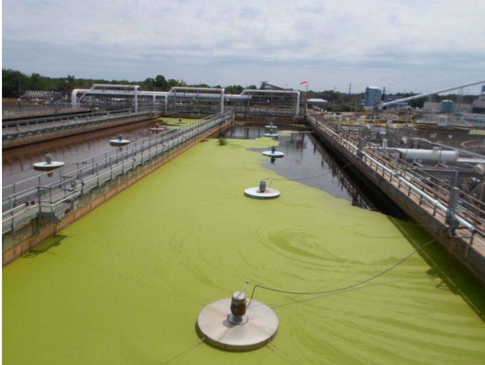
Photograph 32. Duck weed covering approximately 50% of Cell A of tertiary aerator AE-251, which was out of service, at the WWTP.
