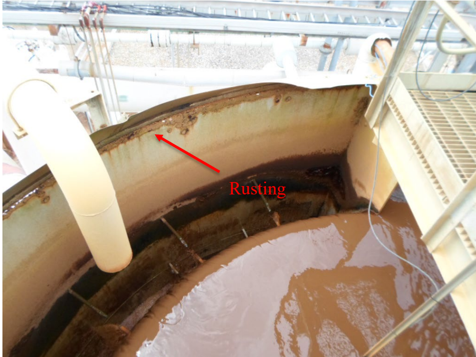
Photograph 23. Flow splitter GT 161 receiving flow from the WWTP's secondary treatment aerators. The structural supports between the exterior wall and internal flow receiver had failed at multiple locations due to rust.
