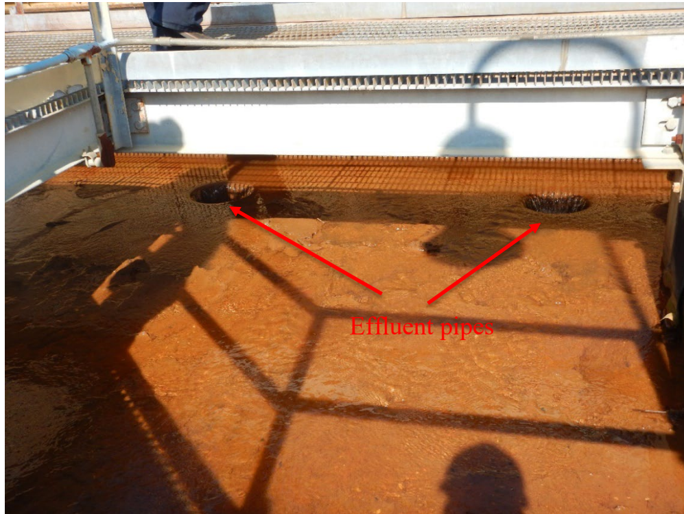
Photograph 17. Solids buildup in the flocculator FL-62, reaching the top of the effluent pipes at the WWTP.
