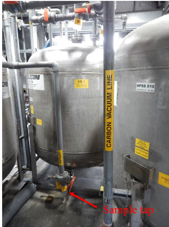
Photograph 56. Sample point for effluent from DuPont's lag GAC bed in the pretreatment system.
