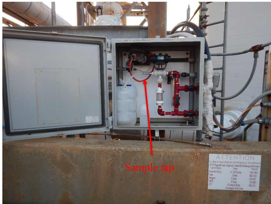
Photograph 44. Sampling box for A Regional Tank.
