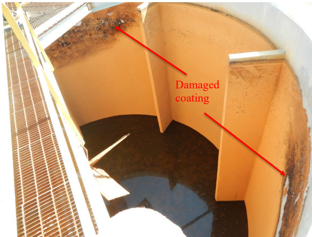
Photograph 20. Damaged coating on the interior of neutralizer NE-43 at the WWTP.
