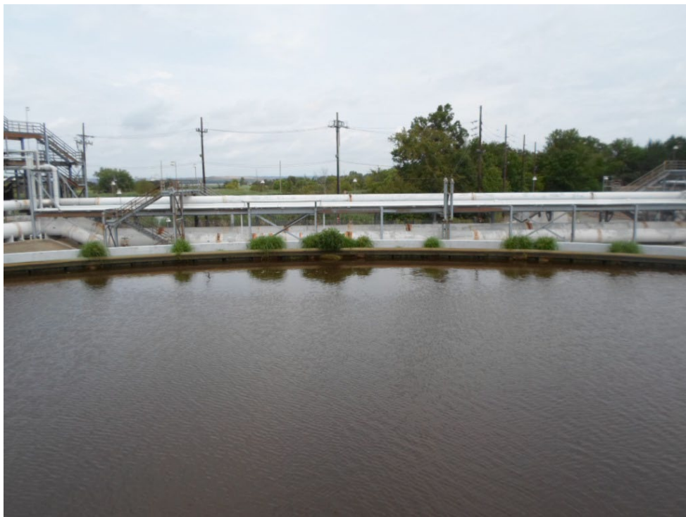
Photograph 30. Vegetation in the effluent trough in multiple locations around secondary clarifier-CF 163 at the WWTP. The process wastewater level was below the weir plate and slowly rising.
