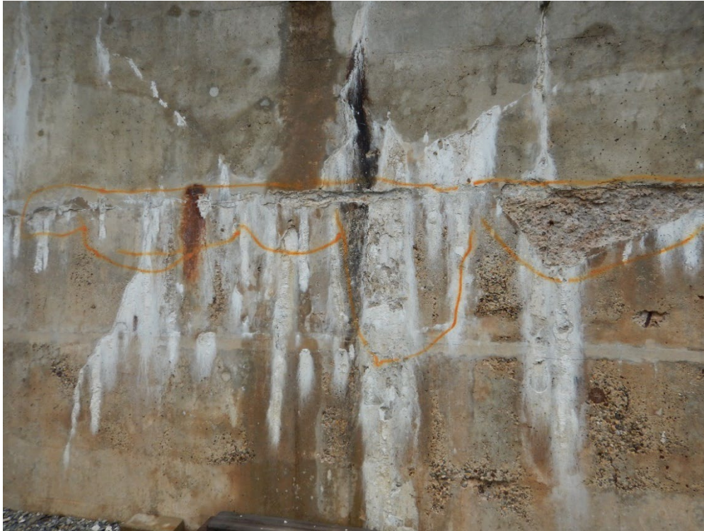
Photograph 5. Cracks, crumbling, and lime (white substance) leaching from the exterior of the WTP clarifier. Note orange outline from previous integrity assessment by outside vendor.
