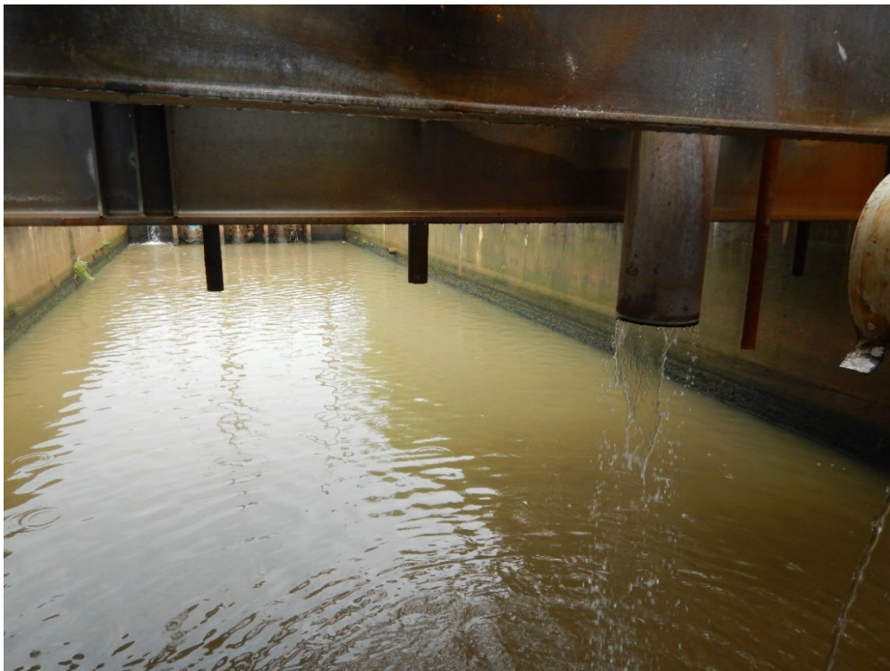
Photograph 10. Sanitary service water bleeding from the sanitary service line distribution pumps into A Basin (which is routed to the WWTP).
