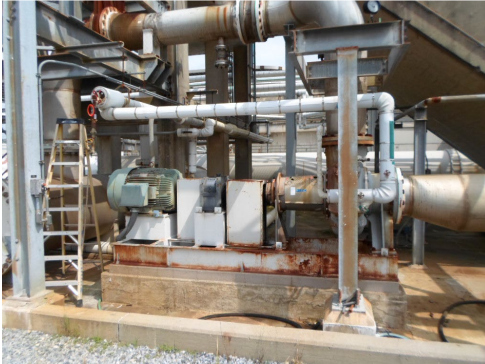
Photograph 39. Pump installed to replace the two screw pumps (pictured above) for returning activated sludge at the WWTP.
