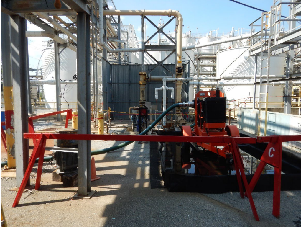
Photograph 37. Temporary pump being used to replace a broken pump used to transport water into the neutralizers at the WWTP.
