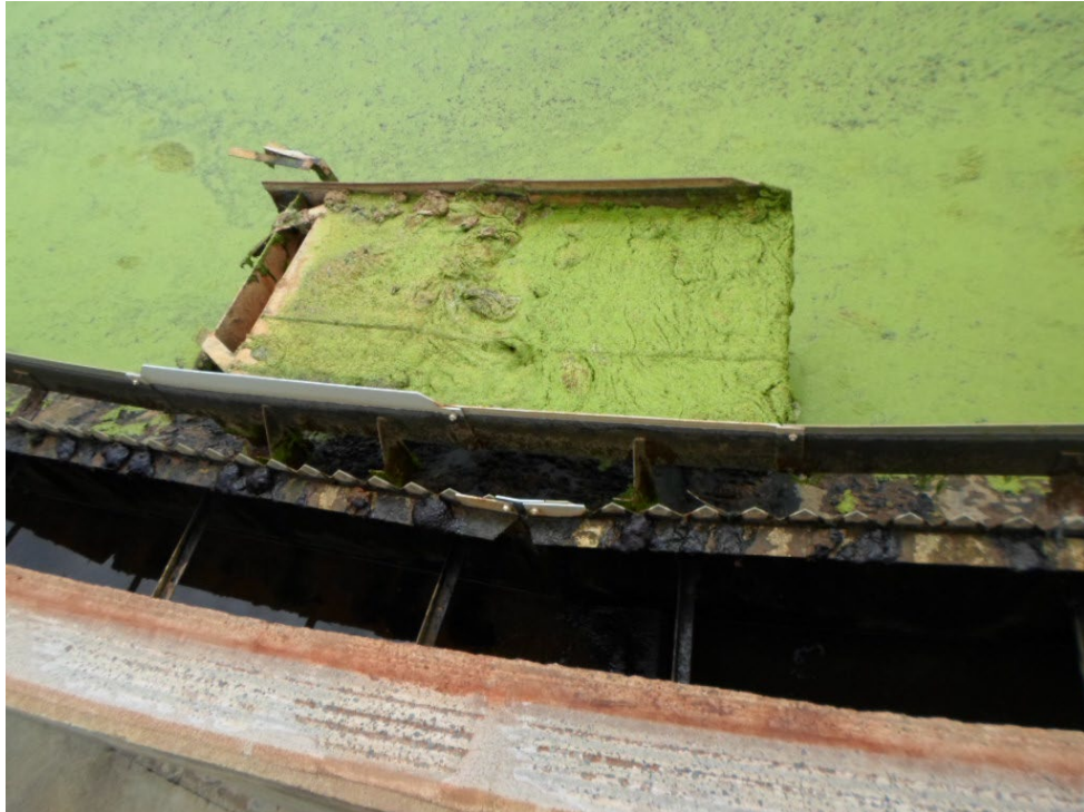
Photograph 29. Alternate view of the duck weed in secondary clarifier CF-162 at the WWTP. The water level was approximately two feet below the weir plate and scum beach due to operational redirection of flows earlier in the day.
