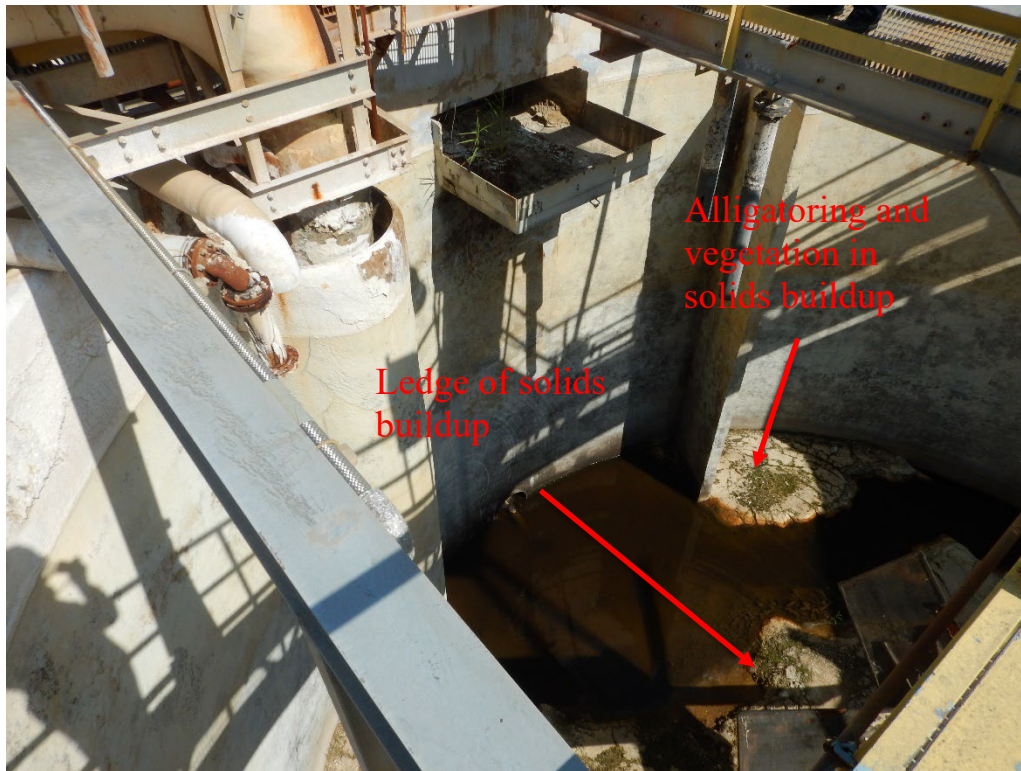
Photograph 13. Alligatoring and vegetation on bottom of the neutralizer NE-41 at the WWTP.
