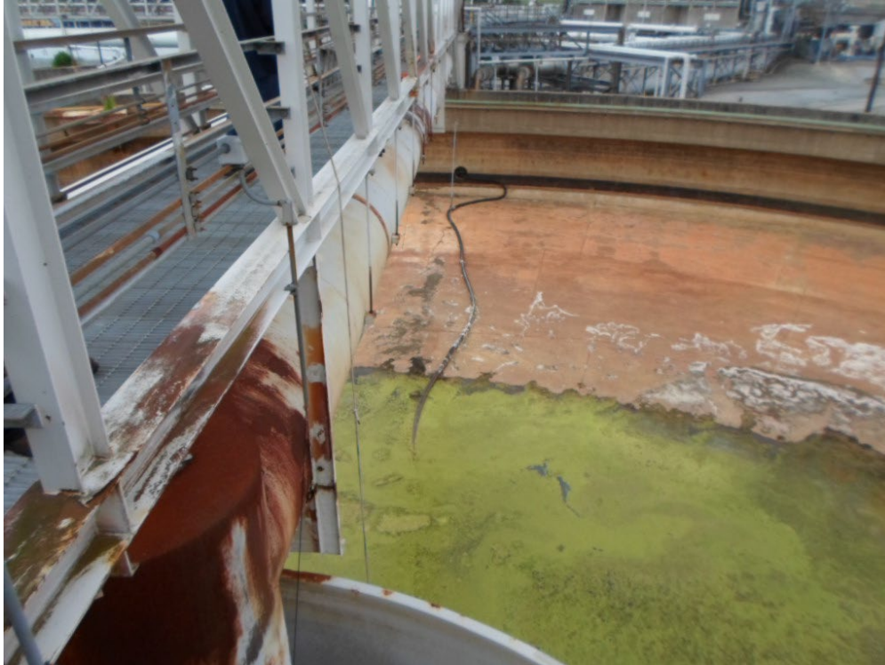
Photograph 34. Vegetation in tertiary clarifier CF-261 at the WWTP. Note CF-261 was out of service and being pumped down with a hose and a Godwin trailered pump.
