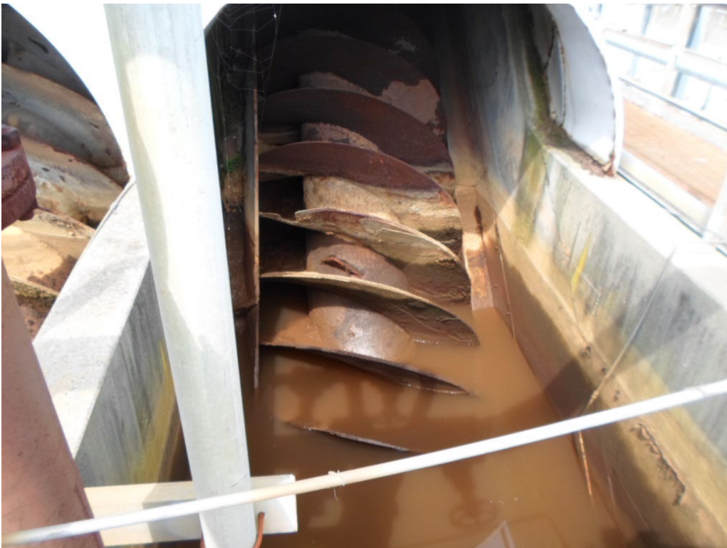
Photograph 38. Decommissioned return activated sludge screw pumps at the WWTP.
