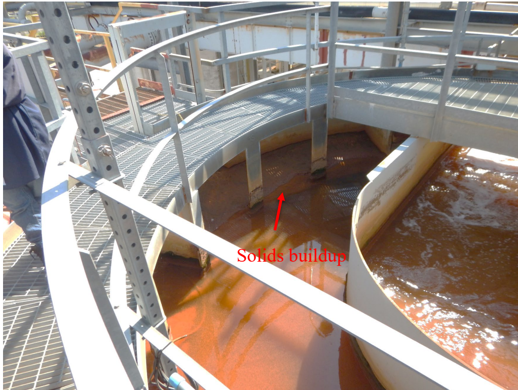
Photograph 15. Solids buildup along outer wall of the flow splitter at the WWTP.
