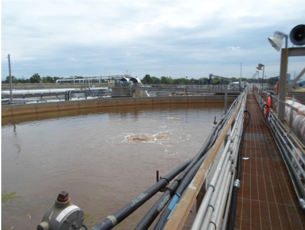
Photograph 11. Aerator AE-153 at the WWTP, which was said to be out of service. The facility was filling the tank during the inspection, thereby decreasing flows through the remainder of the WWTP.
