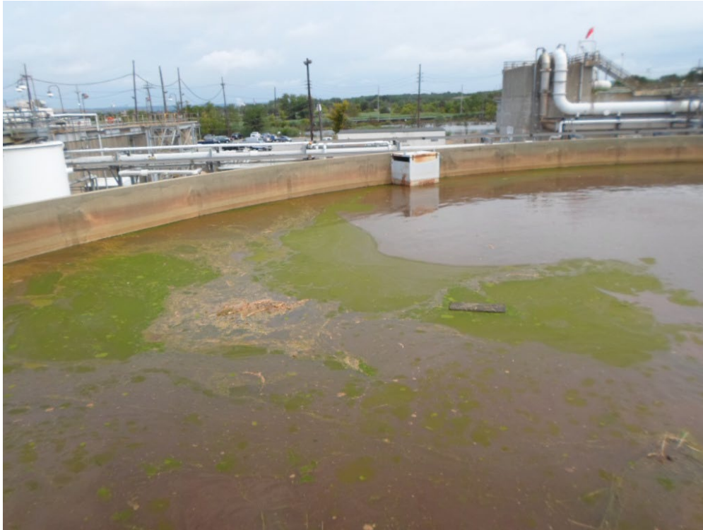
Photograph 27. Secondary treatment aerator AE-153 at the WWTP, with floating debris and vegetation along the surface of the tank.
