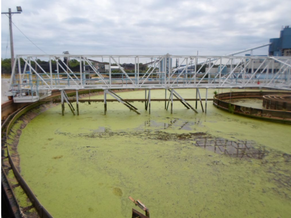
Photograph 28. Secondary clarifier CF-162 at the WWTP, covered with duck weed. Note the clarifier had just started receiving flow from the secondary aeration tanks at the time the photograph was taken.
