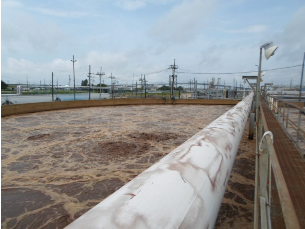
Photograph 40. Secondary treatment aerator AE-152 at the WWTP. Note some areas had excessive air flow.
