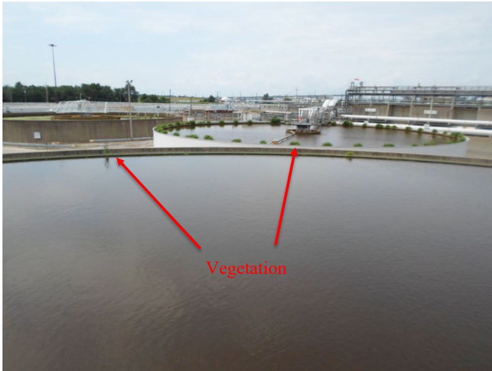
Photograph 35. Vegetation in the effluent trough in multiple locations around tertiary clarifier CF-262 (foreground) and secondary clarifier CF-163 (background) at the WWTP.
