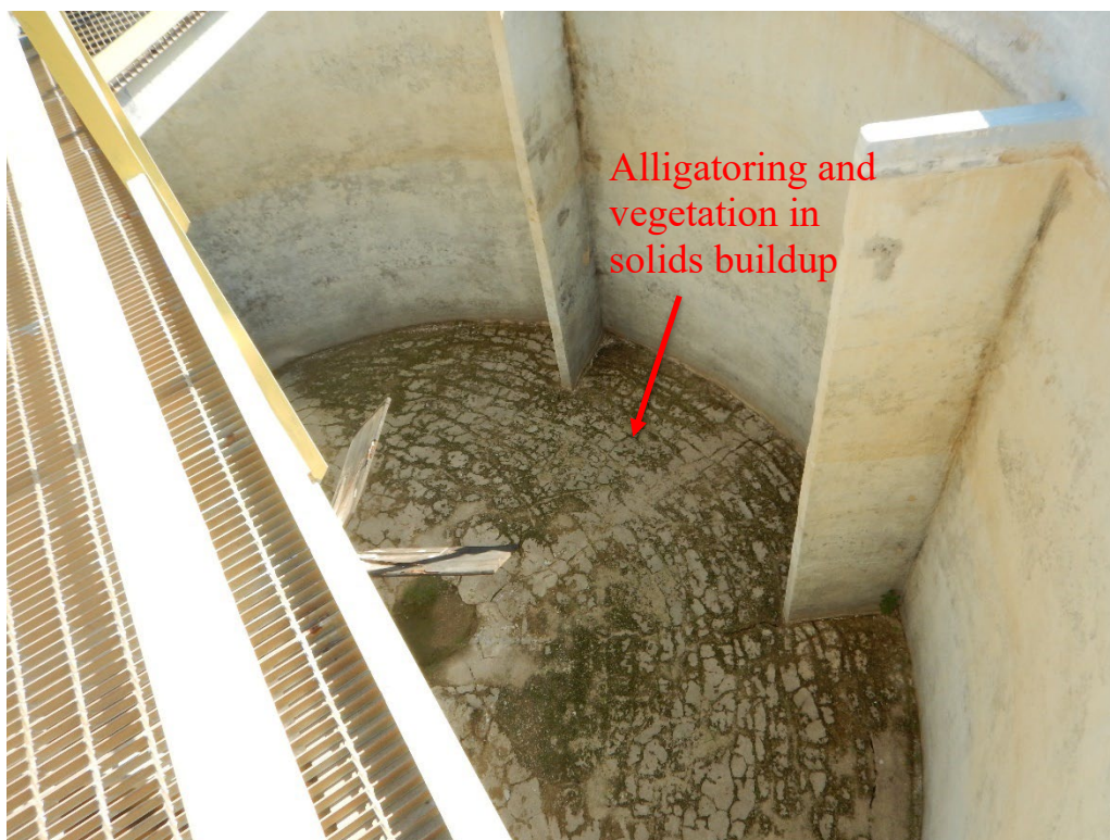
Photograph 14. Alligatoring along bottom of the neutralizer NE-41 at the WWTP.
