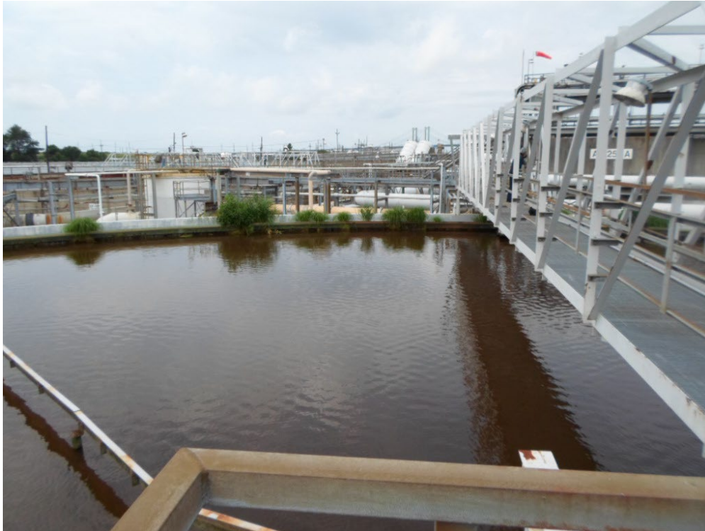
Photograph 31. Alternate view of vegetation in the effluent trough in multiple locations around secondary clarifier-CF 163 at the WWTP. Some vegetation was over four feet high.
