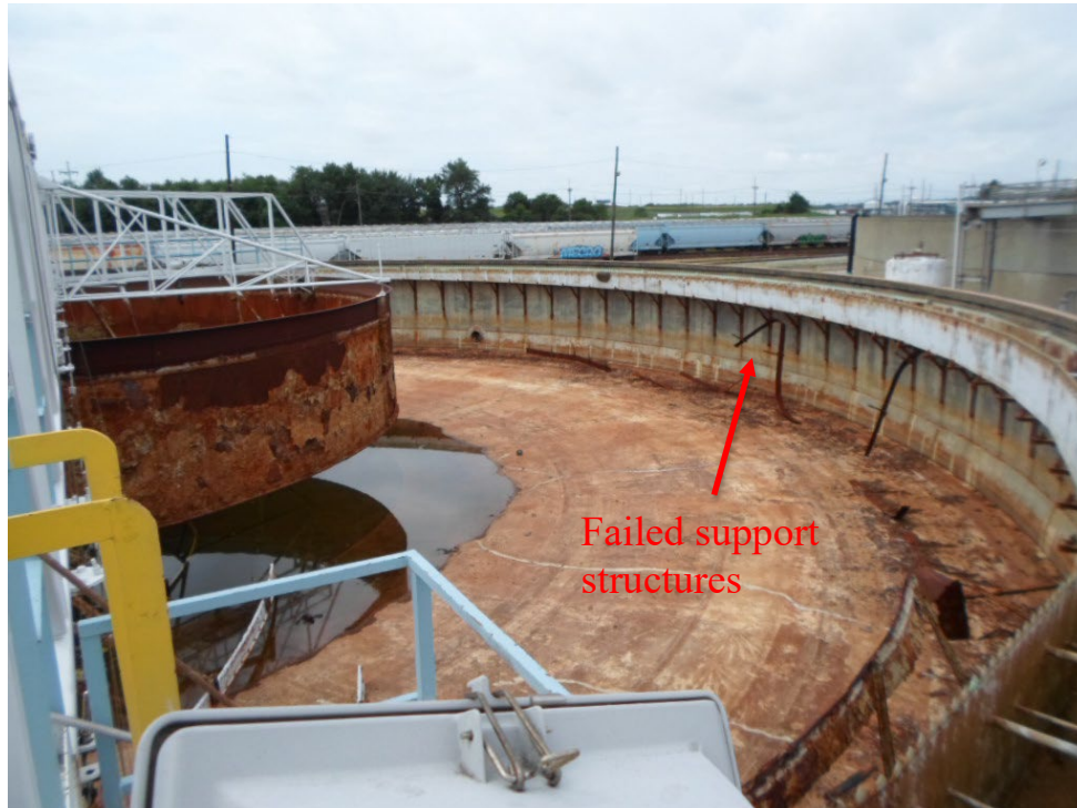
Photograph 25. Secondary clarifier CF-161 at the WWTP, which was out of service at the time of the inspection. The structure supports under the effluent trough had failed and were laying on the bottom of the clarifier and hanging from the trough.
