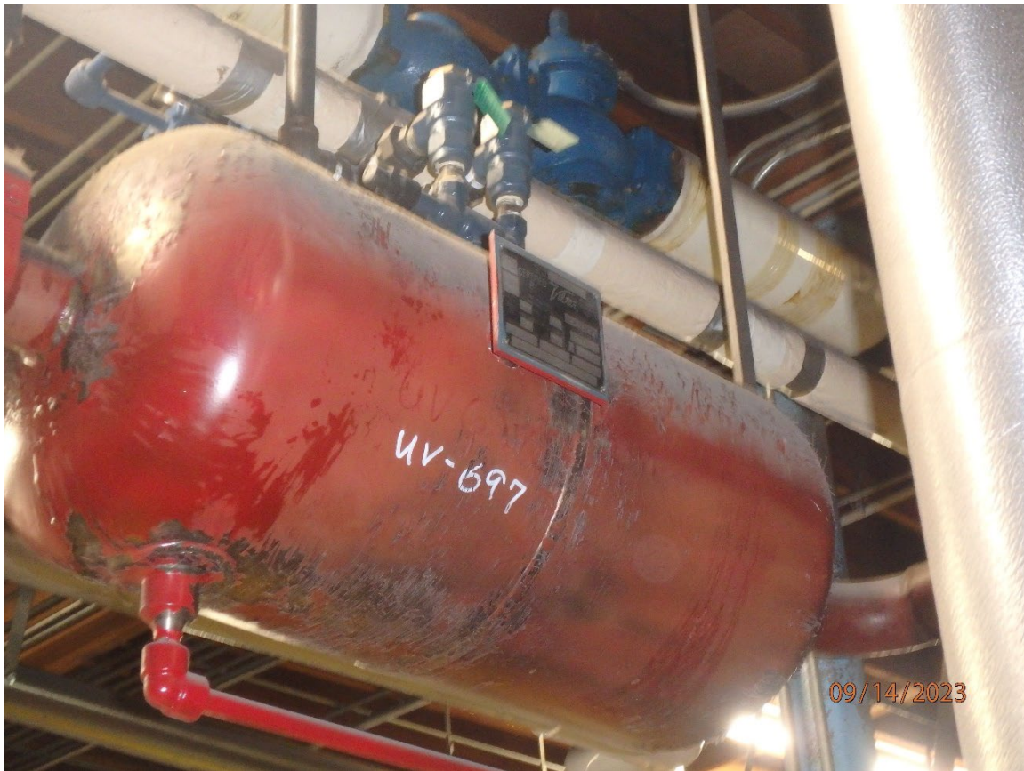
Photo 2. UV-697 visible corrosion
