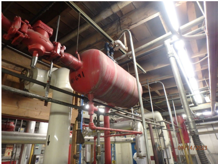
Photo 3. UV-691 visible corrosion
