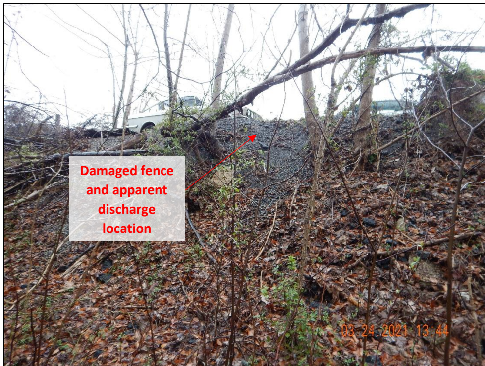
DSCN2237. View, facing north, of a location along the Facility's southwestern perimeter where the fence was damaged and there were signs of discharge.
