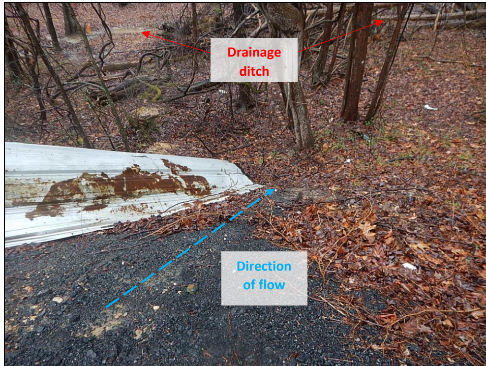
DSCN4081. View, facing south, of a damaged location at the southwestern fence. Evidence of discharge from the Facility was observed at the location.
