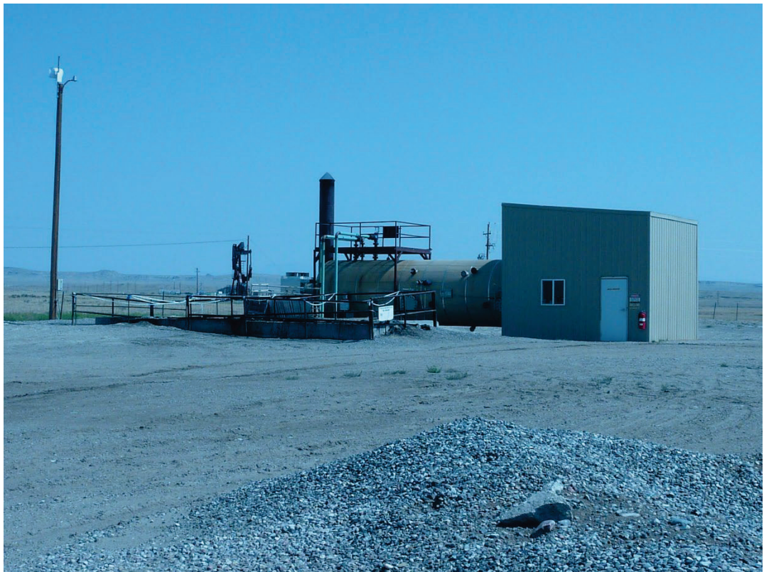
Photo of the Heater Treater
