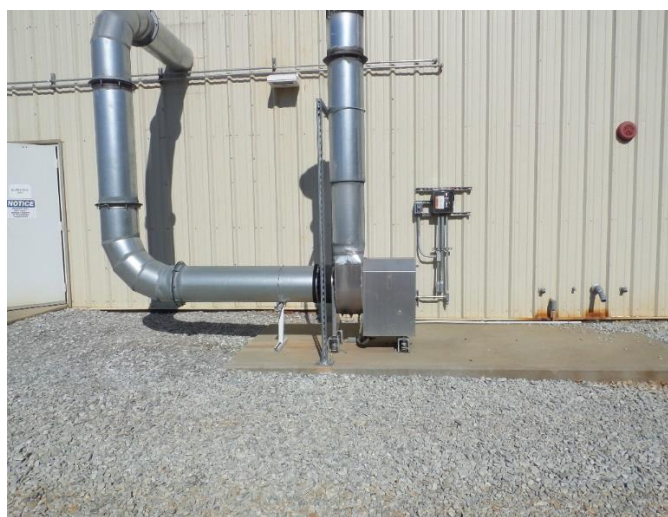
Slurry Building Outdoor Vent System. The inspector observed a ventilation system to exhaust emissions from the distillation units. Photograph 9 taken at 11:13 a.m.
