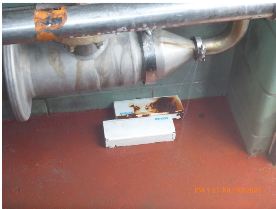
Photograph 3: Gasket on pipe leaking at United Dairy.
