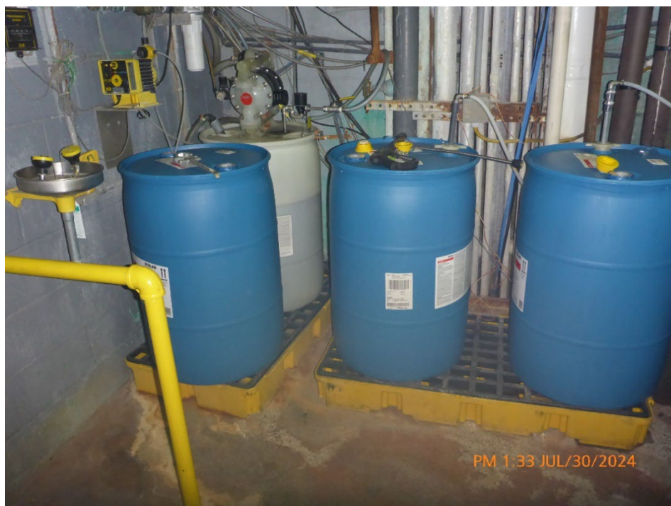
Photograph 2: CIP3 chemical partially on secondary containment pallet at United Dairy.
