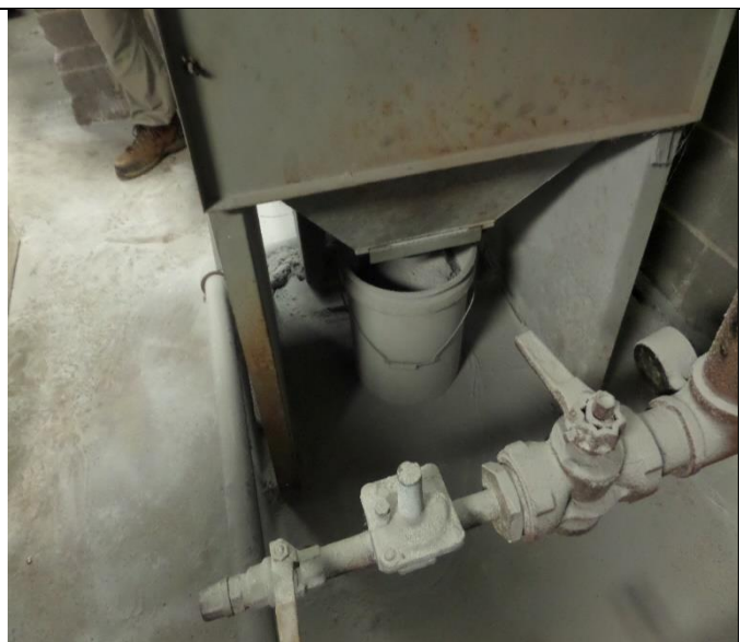
Blast Cabinet Area. Inspectors observed spent blast media in an open 5-gallon container and on the floor. The blast cabinet was not operating. Photograph 3 taken at 10:13 a.m.
