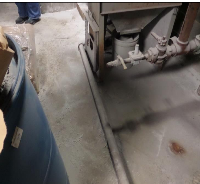
Blast Cabinet Area. Inspectors observed spent blast media in an open 5-gallon container and on the floor. Photograph 4 taken at 10:14 a.m.
