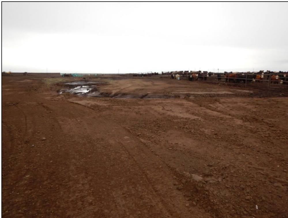
Photograph 12. Settling cell SC-12 receives runoff from adjacent cattle pens, view looking east.
