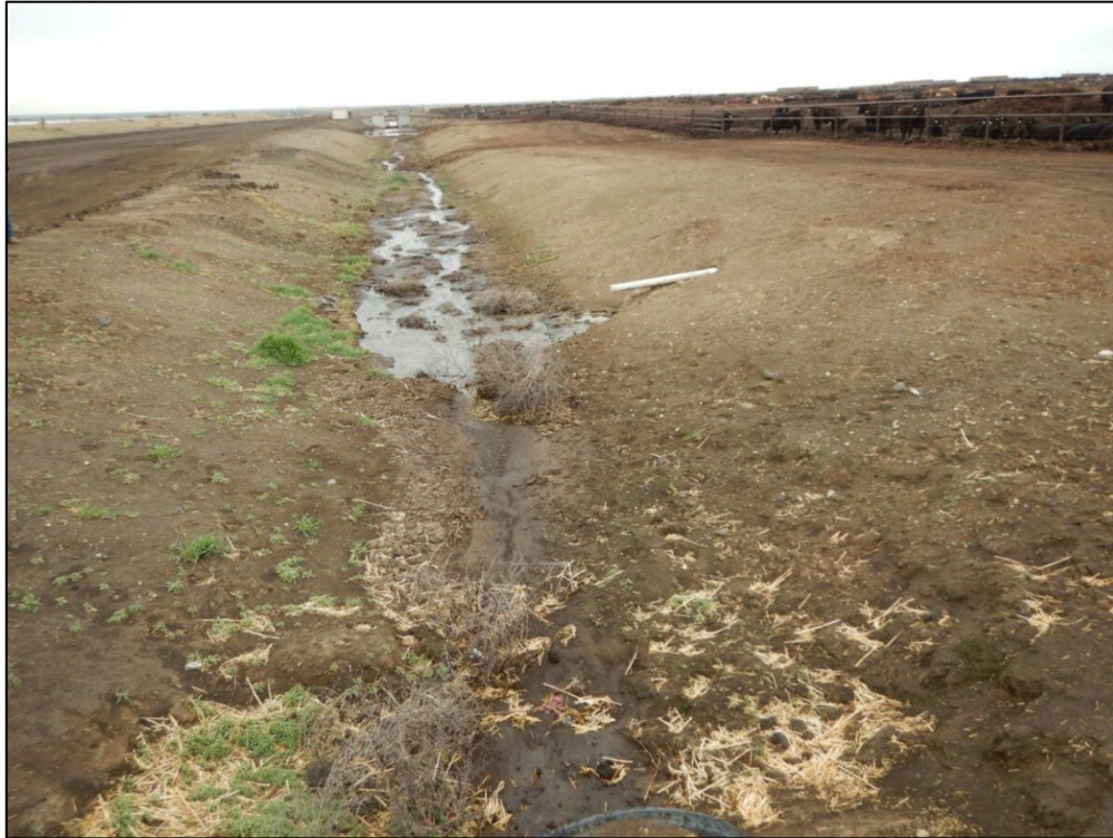
Photograph 15. Conveyance ditch CD-2b conveys cattle pen runoff to settling cell SC-14, view looking east.
