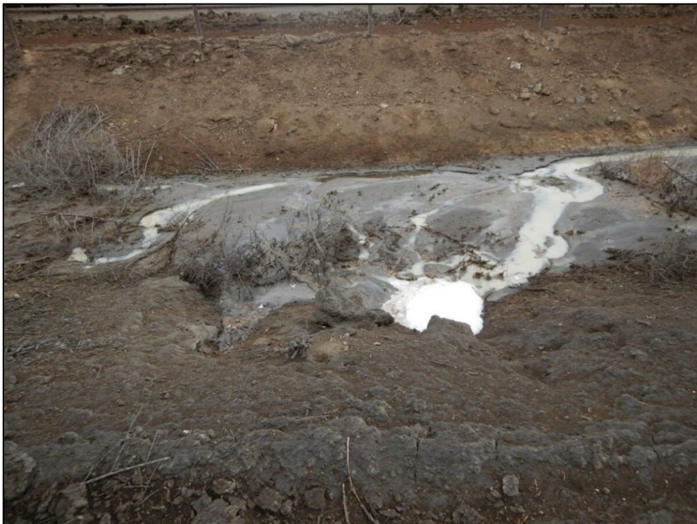
Photograph 28. View of point in conveyance ditch CD-3 where wastewater from the mill and boiler blow down enter the ditch. Conveyance ditch CD-3 flows south to settling cell SC-7 and then to a pump station which pumps wastewater to Lagoon 1.
