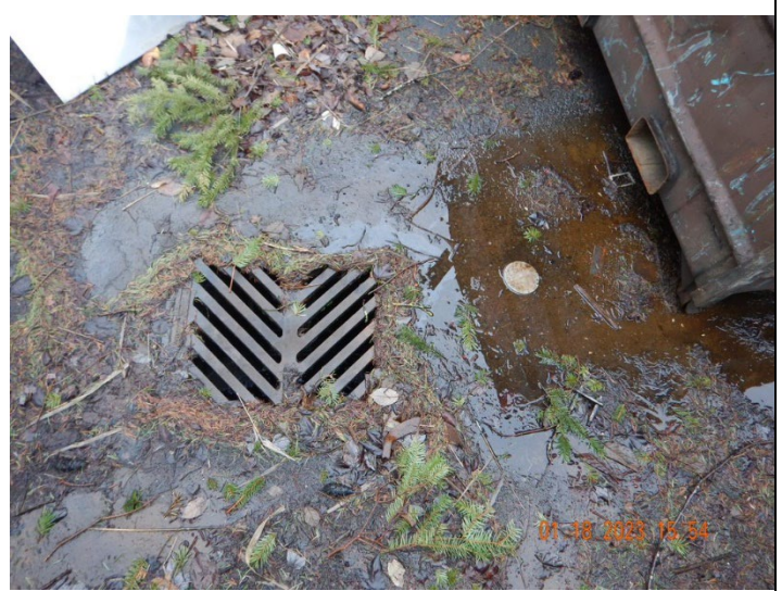
Photo #:12 (DSCN0538) Description: Facing east, photo of a catch basin next to the open roll-off in previous photos.
