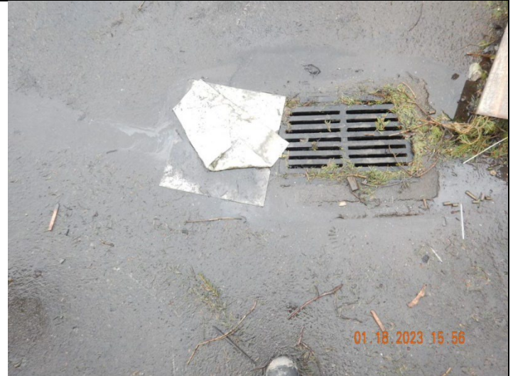
Photo #: 16 (DSC0542) Description: Facing east, a second catch basin with absorbent pads placed to the side. Stormwater flowing towards catch basin contained a sheen.
