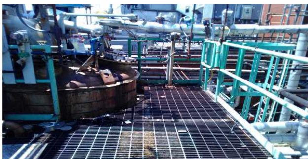
Photo 2: Picture provided May 25, 2021. The two 1-gallon containers observed during the inspection had been removed from the Tank 14/15 catwalk.
