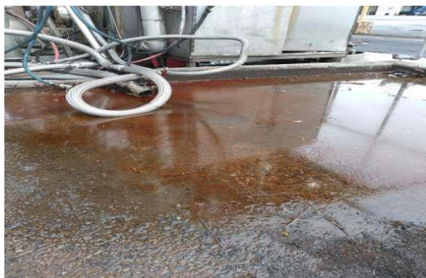
Photo 16: Bldg. 201 dumpster pad. Red tinted water in secondary containment.
