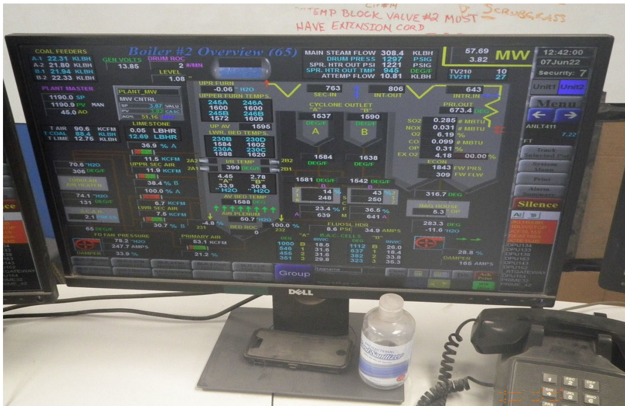
14. Boiler 2 Control Room Overview – Scrubgrass Generating – 6/7/22
