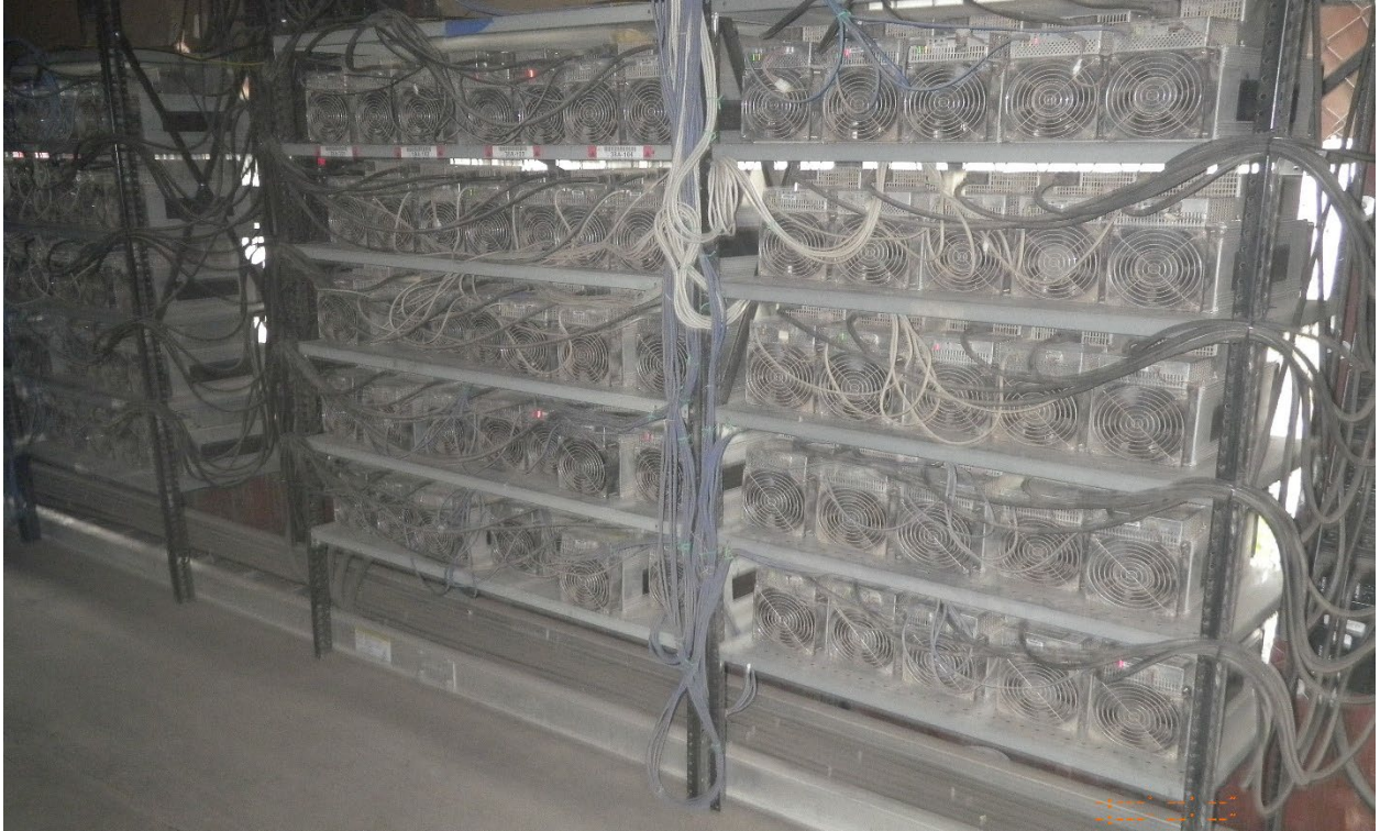
24. Computers Inside Storage Container in Data Center – Scrubgrass Generating – 6/7/22
