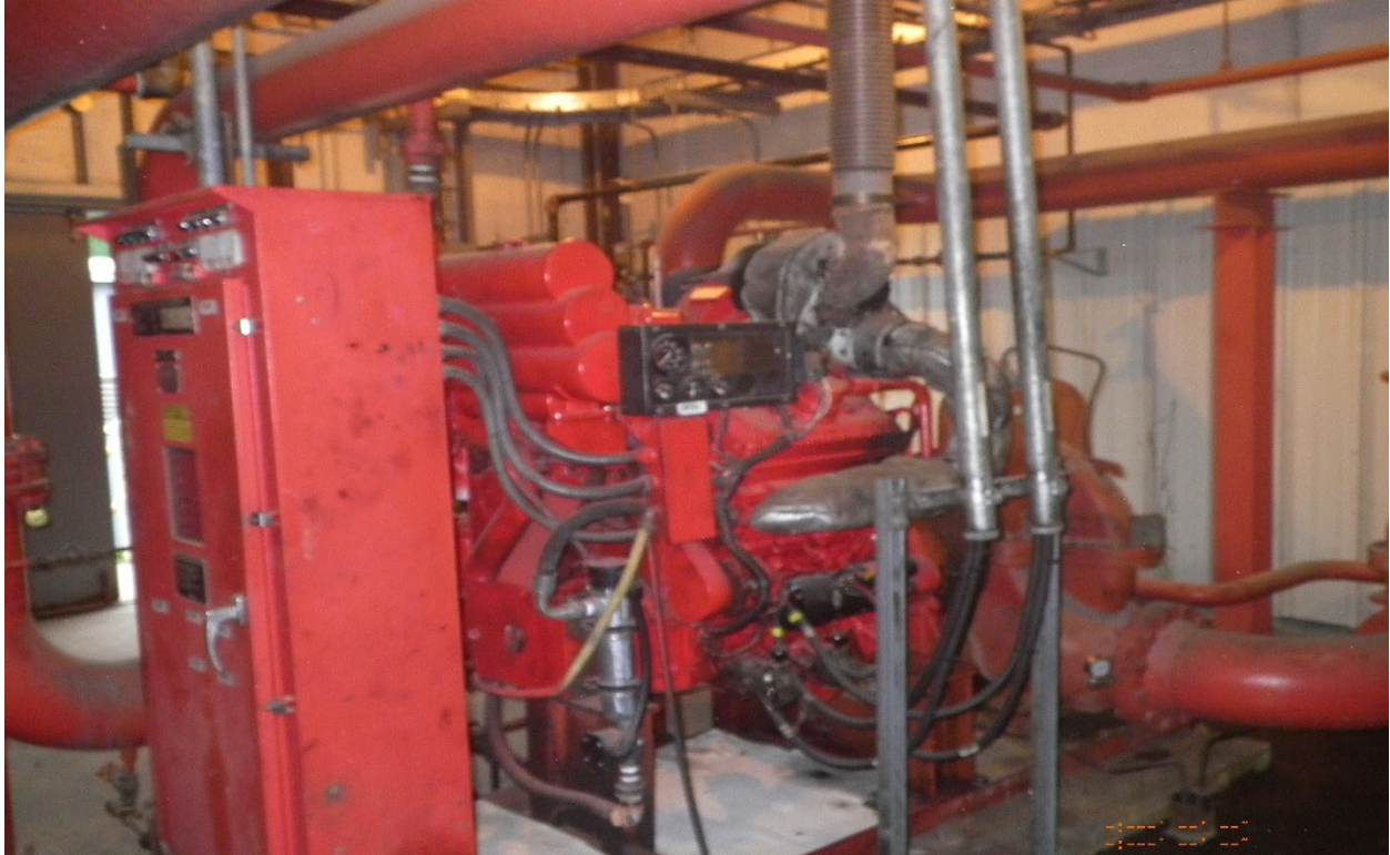
10. Diesel Fire Pump – Scrubgrass Generating – 6/7/22
