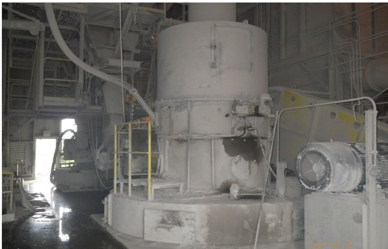
7. Limestone Crusher – Scrubgrass Generating – 6/7/22
