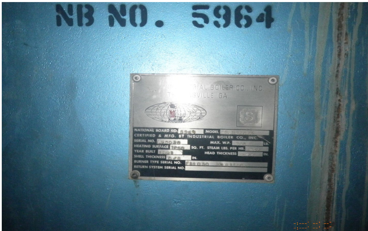
9. Auxiliary Boiler Nameplate – Scrubgrass Generating – 6/7/22
