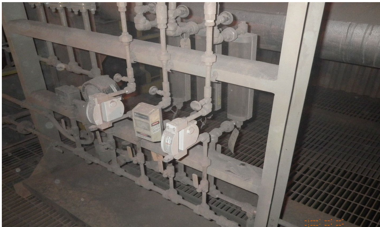
20. Ammonia Injection Piping and Flow Meter – Scrubgrass Generating – 6/7/22
