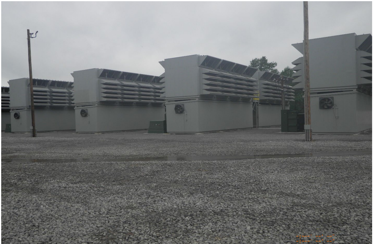
25. New Design Computer Containers at Data Center – Scrubgrass Generating – 6/7/22
