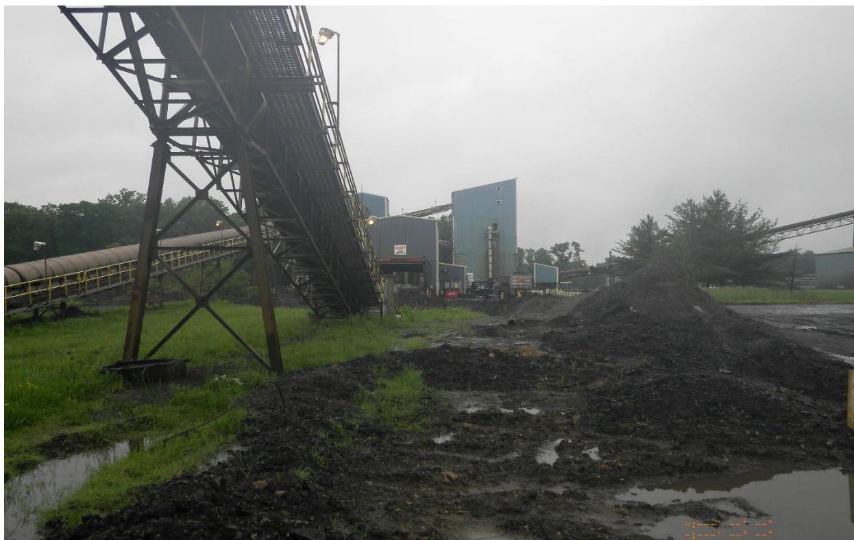
2. Conveyor & Coal Drop Building for Coal Delivery – Scrubgrass Generating – 6/7/22
