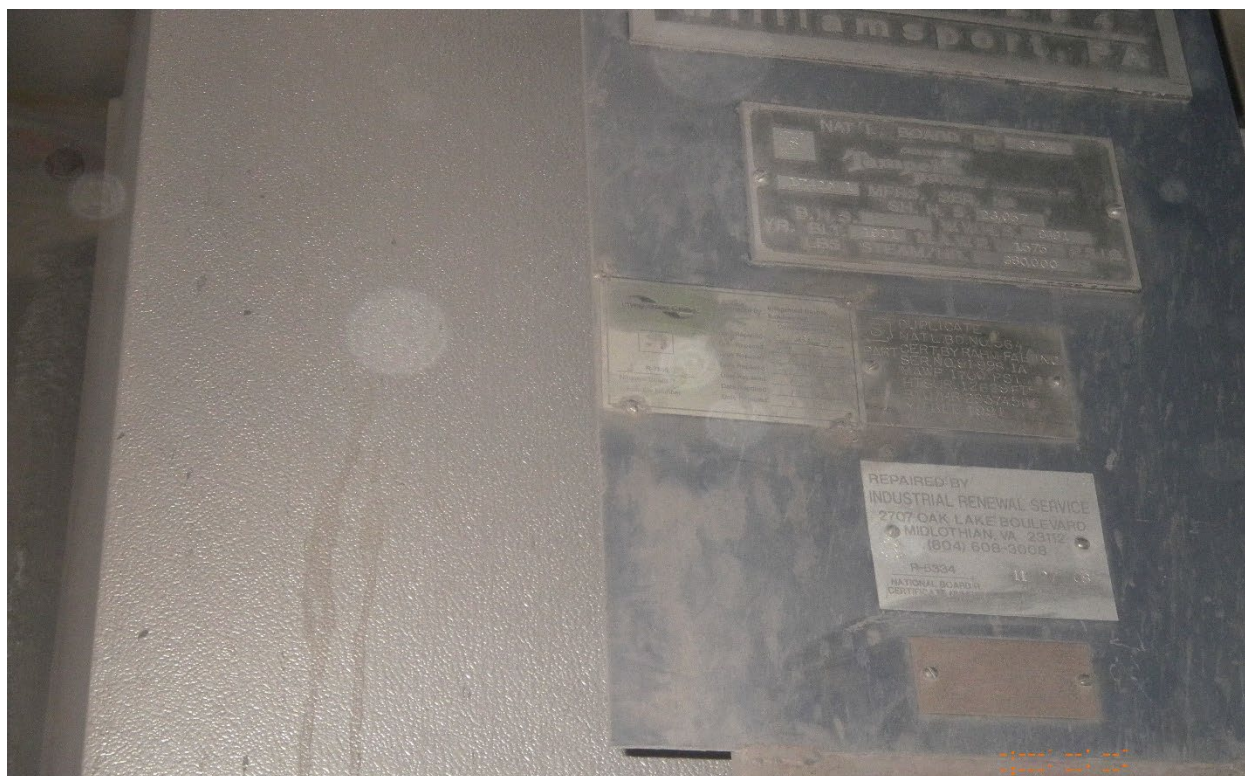
18. Boiler 1 Nameplate – Scrubgrass Generating – 6/7/22
