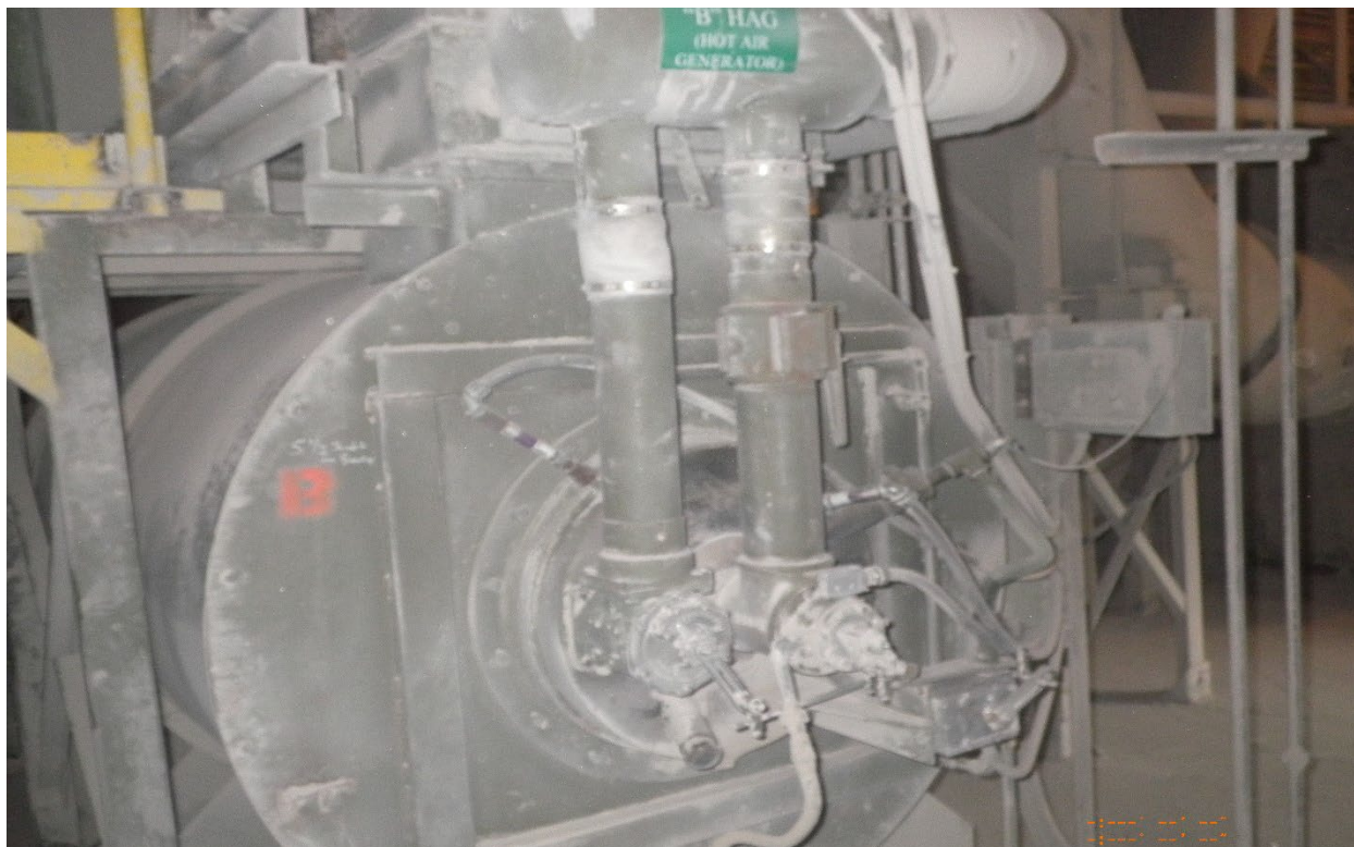
6. Hot Air Generator for Limestone Drying – Scrubgrass Generating – 6/7/22
