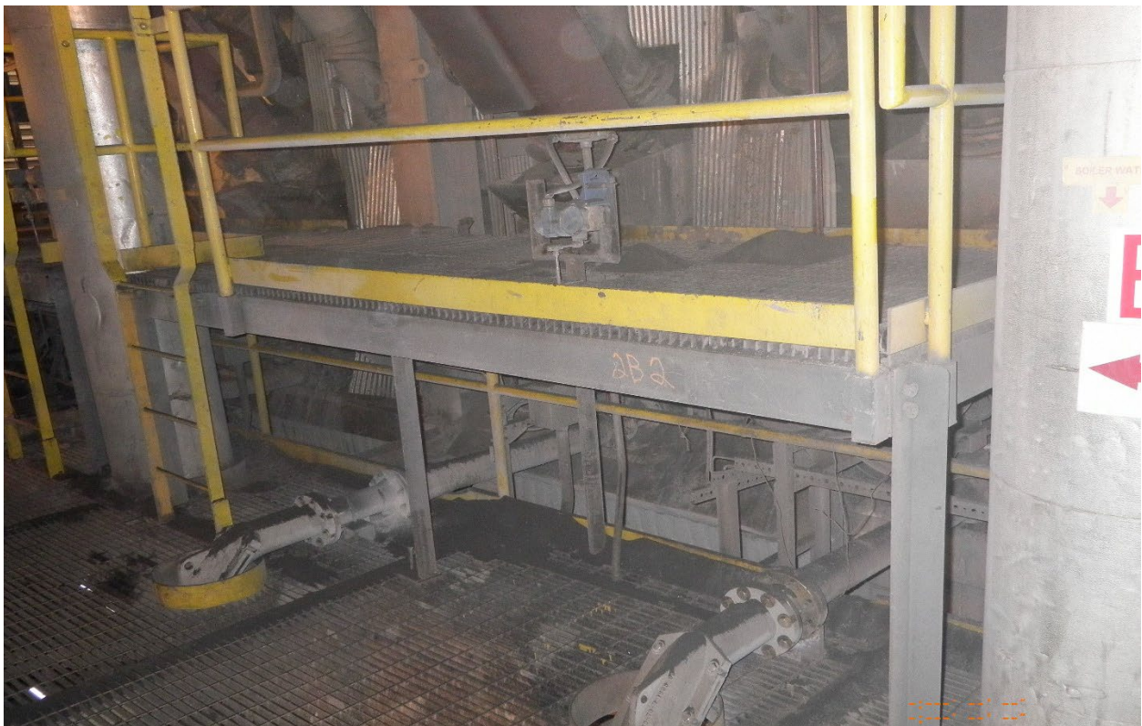
11. Coal and Limestone Injection Points Boiler 2 – Scrubgrass Generating – 6/7/22
