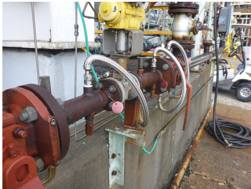
Photo 6: Equipment tags to identify Tank 8T018 ancillary equipment that is subject to air monitoring under RCRA Subpart BB.
