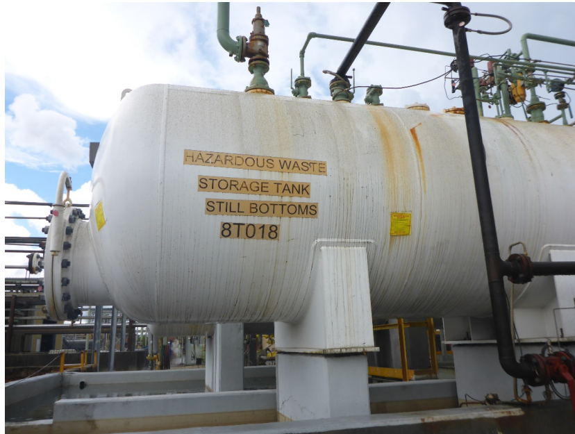
Photo 5: 5,000-gallon hazardous waste storage tank, Tank 8T018.
