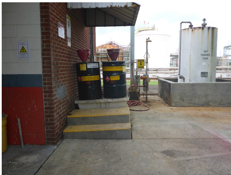
Photo 1: Two SAAs in the Paint Shop Area. One SAA is used to accumulate hazardous waste paint thinner as D001, F003, F005 hazardous waste flammable liquid (toluene, methanol), the other is used to accumulate hazardous waste paint solids as D001, F003, F005 hazardous waste paint related material.
