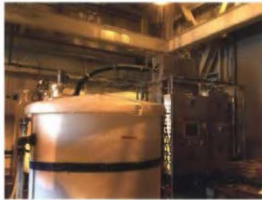
Figure 3-2 ZeeWeed 500 MBR pilot Courtesy of GE Water & Process Technologies
