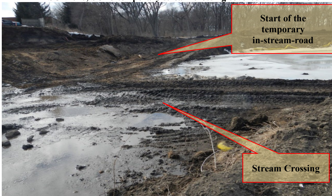
DSCN1070, SC #3 temporary stream crossing covered with sediment
