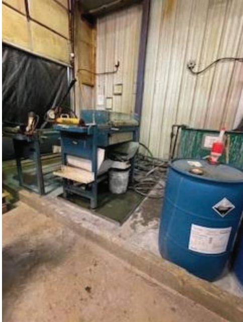
Photo 18: Photo of the wastewater treatment filter press.
