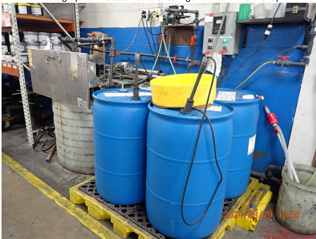
Photograph 7: Chemical storage at RR Donnelley.
