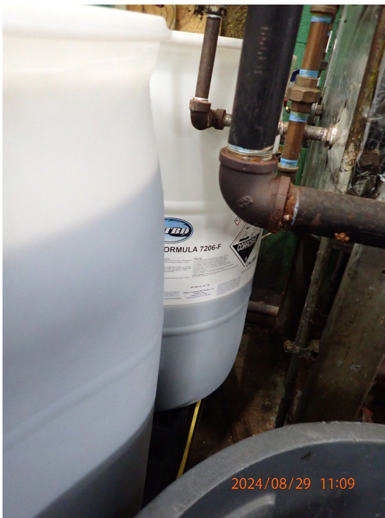
Photograph 9: Drum hanging off of the secondary containment pallet at RR Donnelley.
