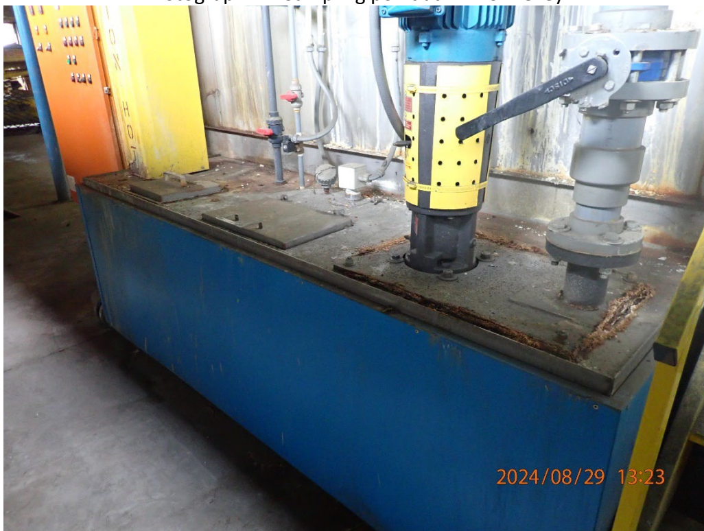
Photograph 13: Powder coating tanks used for rinses at Lepko.
