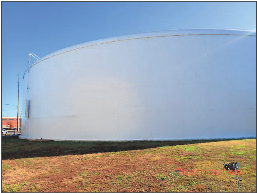
Photograph 2. 11/20/2024 14:06 Description: I Street 6-MG Tank located on the same site as the I Street Pump Station.
