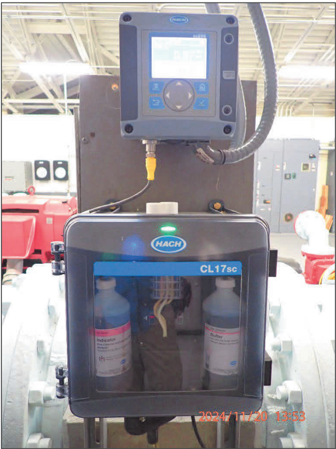
Photograph 3. 11/20/2024 13:53 Description: I Street Pump Station. Chlorine residual is monitored at the pump station to confirm an adequate residual from Beaver Water District.
