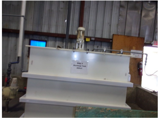
Photo 6: Building #9, 1,200-gallon tank in secondary containment
