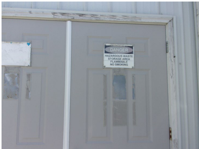
Photo 13: CAA Faded/unreadable labels
