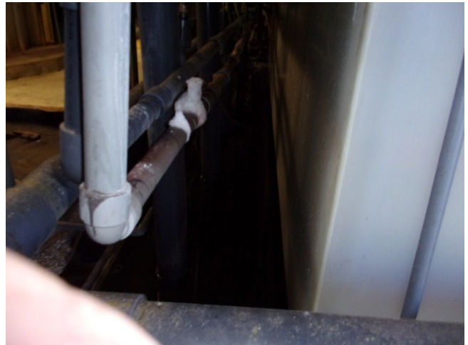
Photo 4: Building #9, secondary containment for the condensate liquid
