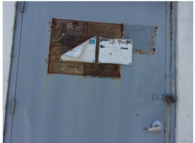
Photo 12: CAA Faded/unreadable labels
