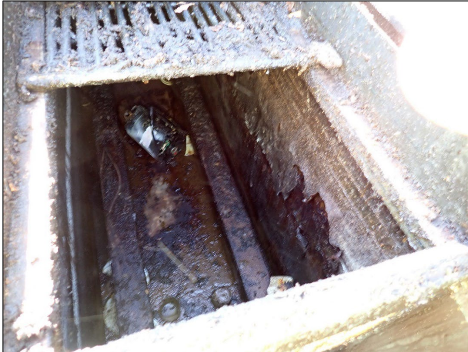
Photograph 3. View of used cooking oil and grease inside one of the containers shown in Photograph 2.
