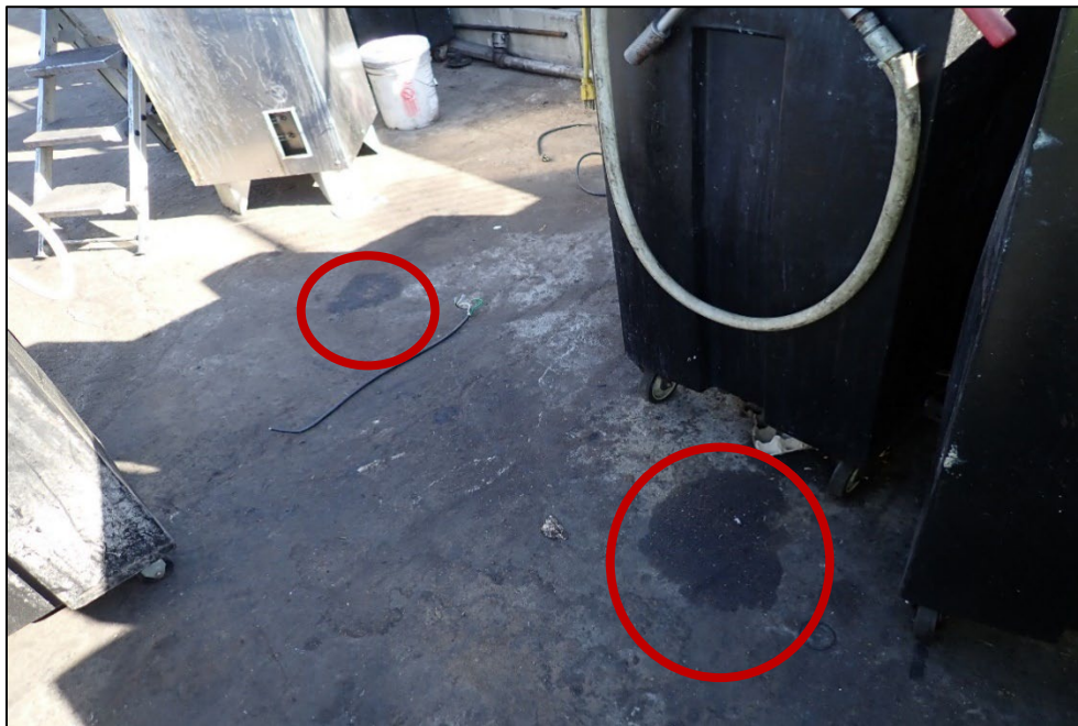
Photograph 8. View of used cooking oil stains on the ground surface in front of an empty used cooking oil container in the eastern portion of the Facility.
