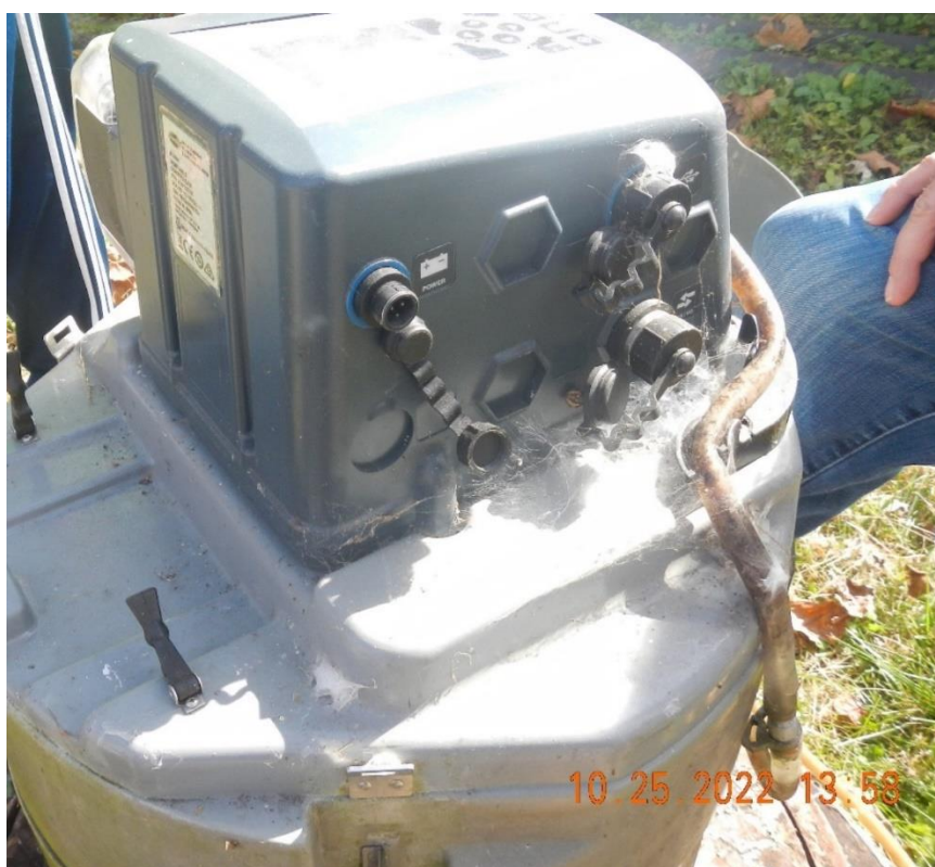
Figure 3. Effluent composite sampler. Suction tube was brittle, broken, and had excessive bacteria lining the interior.
