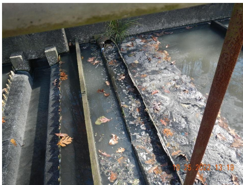
Figure 7. Excessive solids observed floating in the clarifier.
