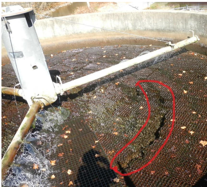
Figure 6. Secondary trickling filter unit. Red lines outline surface damage to the modular plastic media.
