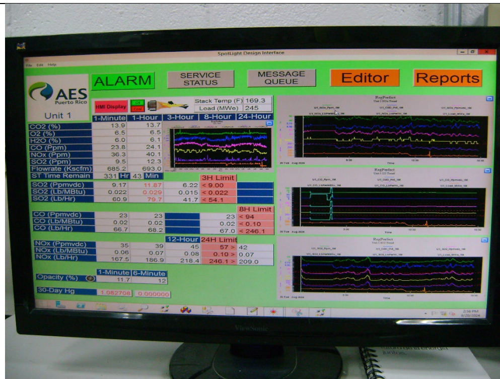
Unit 1 process monitoring screen in CEMS room.
