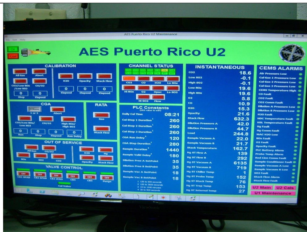
Unit 2 process monitoring screen in CEMS room.
