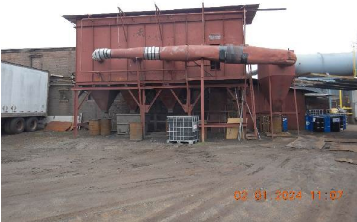
View of the baghouse system connected to the shot blast units, which are inside the building. Spent media and fines are collected in 55-gallon drums and other open-top containers.
