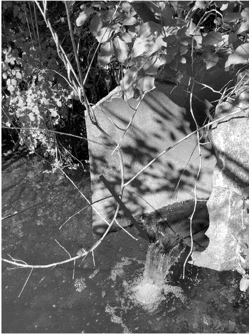
PleasVal (photo taken 5/24 at 09:03 AM): Outfall located on the northeast corner of Chippy Lane and Pleasant Valley St. flowing into Bare Meadow Brook. Sample point is indicated by a red arrow.
