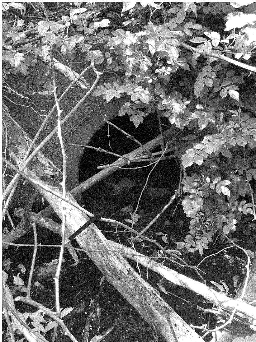
Walton (photo taken 5/24 at 10:18 AM): Close-up view of the outfall where the sample was collected. Sample point is indicated by a red arrow.
