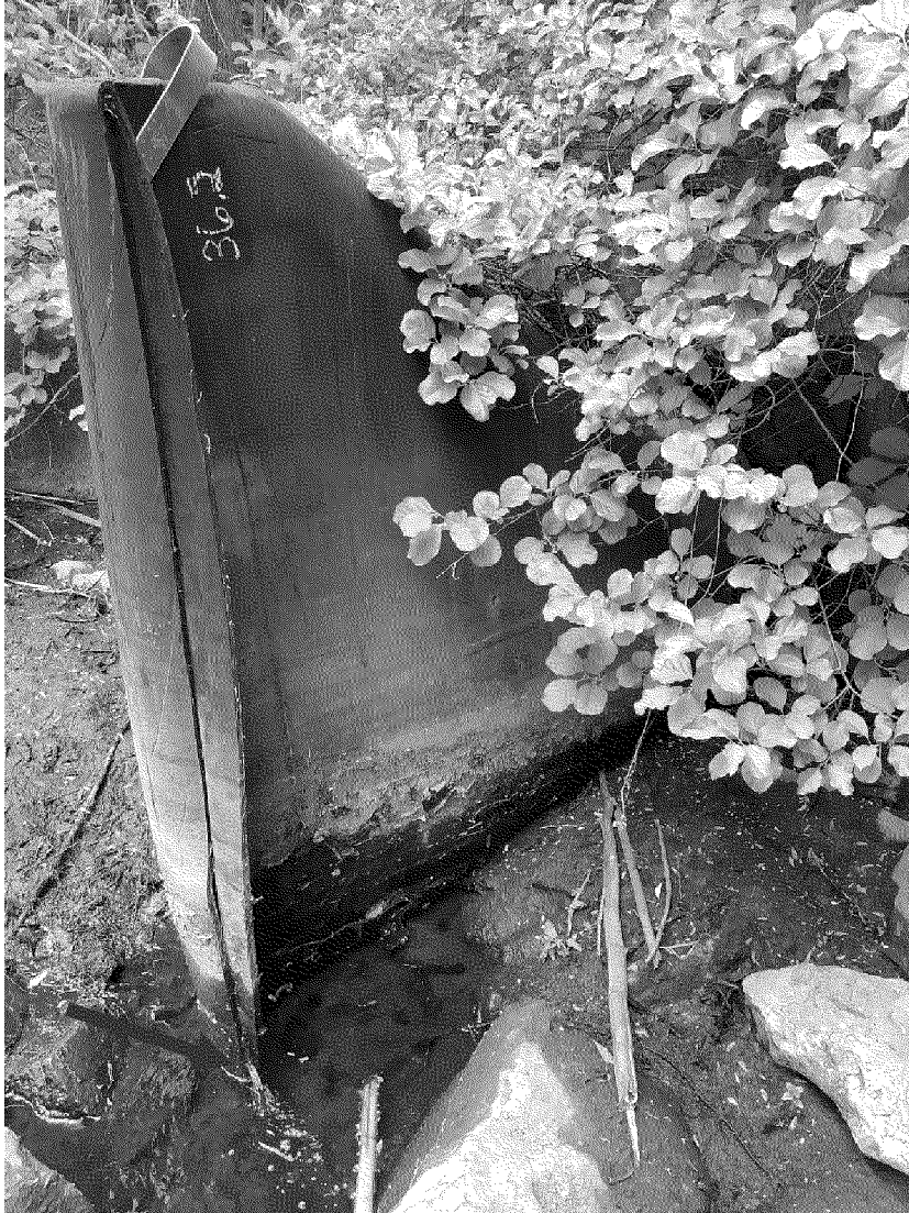
ParkStCVS (photo taken 5/24 at 12:58 PM): Outfall with duckbill located on the southeast corner of the CVS parking lot on Park Street, flowing into the Spickett River. Sample point is indicated by a red arrow.
