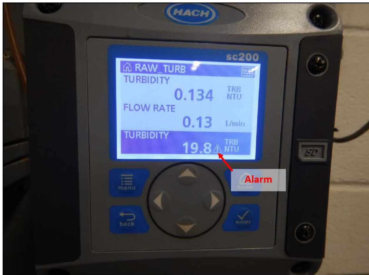
Photograph 16. Turbidity Meter, WTP #01 View of the raw water turbidimeter after the System Manager tried to fix the influent raw water line. The meter was reading 19.8 NTU, and an alarm was still being displayed.
