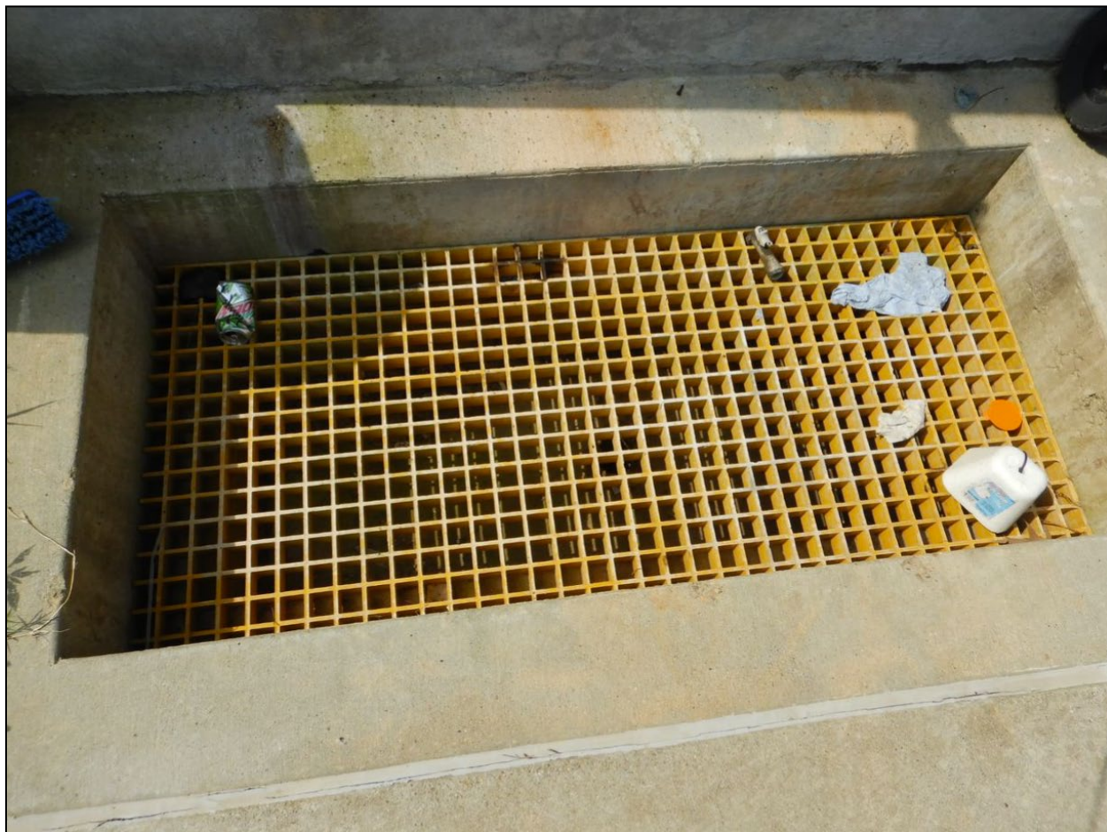
Photograph 7. Chemical Delivery Port Drain, WTP #01 View of the drain positioned below the chemical delivery ports at WTP #01. The System Manager stated that the drain led to an onsite backwash pond. It is unclear if this presents a concern for the plant's NPDES permit.
