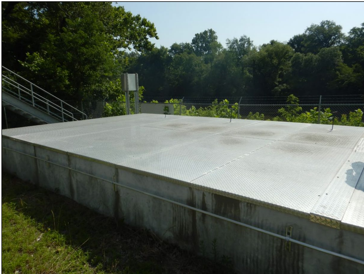
Photograph 4. Raw Water Intake Pumps, WTP #01 View of the vault containing the four, raw water intake pumps next to the Ouachita River at WTP #01.
