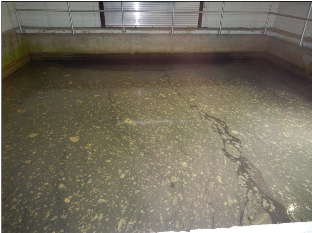
Photograph 18. Filter No. 1, WTP #01 View of the surface of the water in Filter No. 1 at WTP #01. There was a buildup of foam on the surface of the water, and System representatives stated that they may have been over feeding coagulant.
