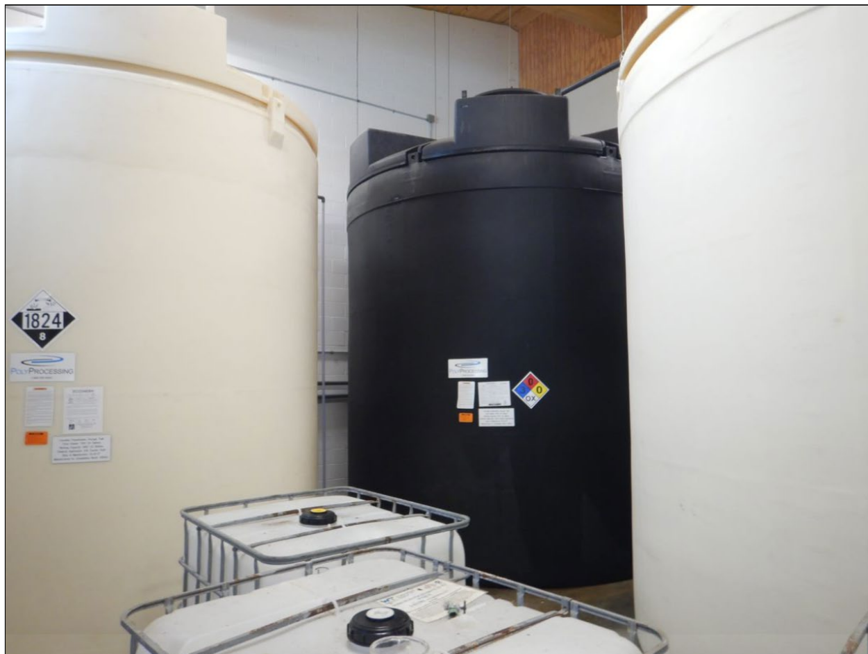
Photograph 13. Chemical Storage Tanks, WTP #01 View of the caustic tank, a sodium hypochlorite tank, and a coagulant tank in the storage area at WTP #01. The tanks were labeled.
