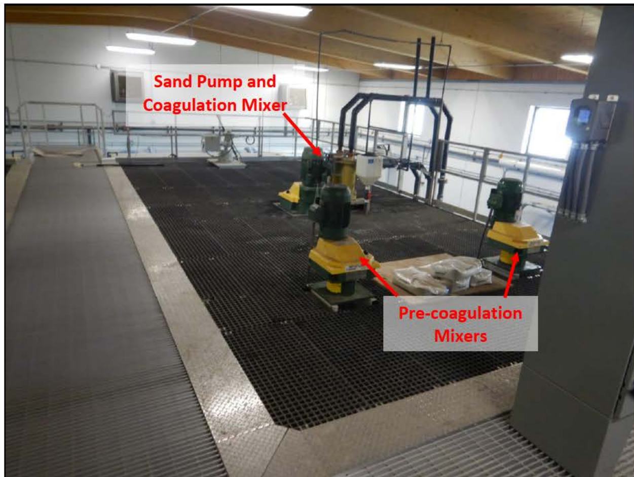
Photograph 17. Treatment Train, WTP #01 View of one of the two parallel treatment trains at WTP #01. Visible in this image are the pre-coagulation mixers, the sand pump, and the coagulation mixers.
