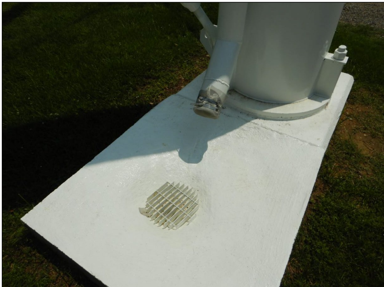
Photograph 37. Overflow Pipe, 16 th St. Water Storage Tank View of the 16 th St. Water Storage Tank overflow pipe. The overflow pipe terminated approximately nine inches above a concrete pad, which appeared to be less than double the pipe diameter.
