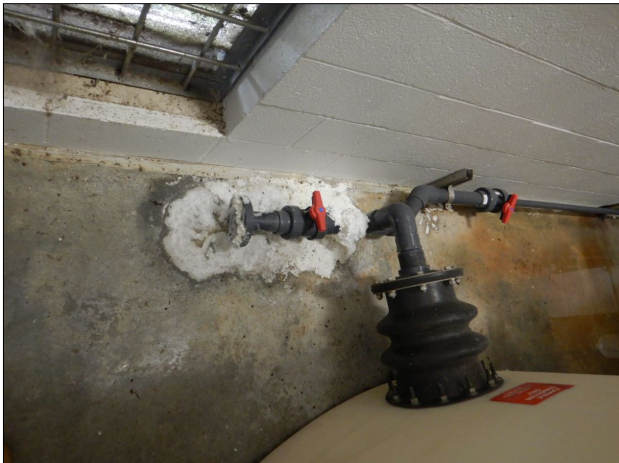
Photograph 14. Caustic Line, WTP #01 View of the line leading to the caustic tank. The line was experiencing a leak and there was crystallized caustic on the ground surrounding the line. The System Manager stated that this happened often, and vinegar was poured on the leak to neutralize it.
