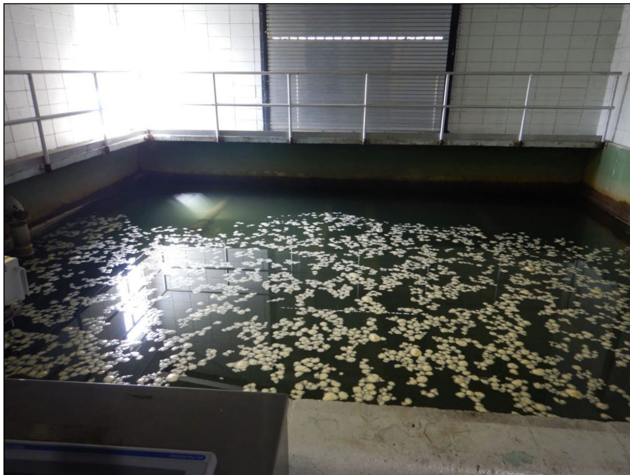
Photograph 19. Filter No. 2, WTP #01 View of the surface of the water in Filter No. 2 at WTP #01. There was a buildup of foam on the surface of the water, and System representatives stated that they may have been over feeding coagulant.
