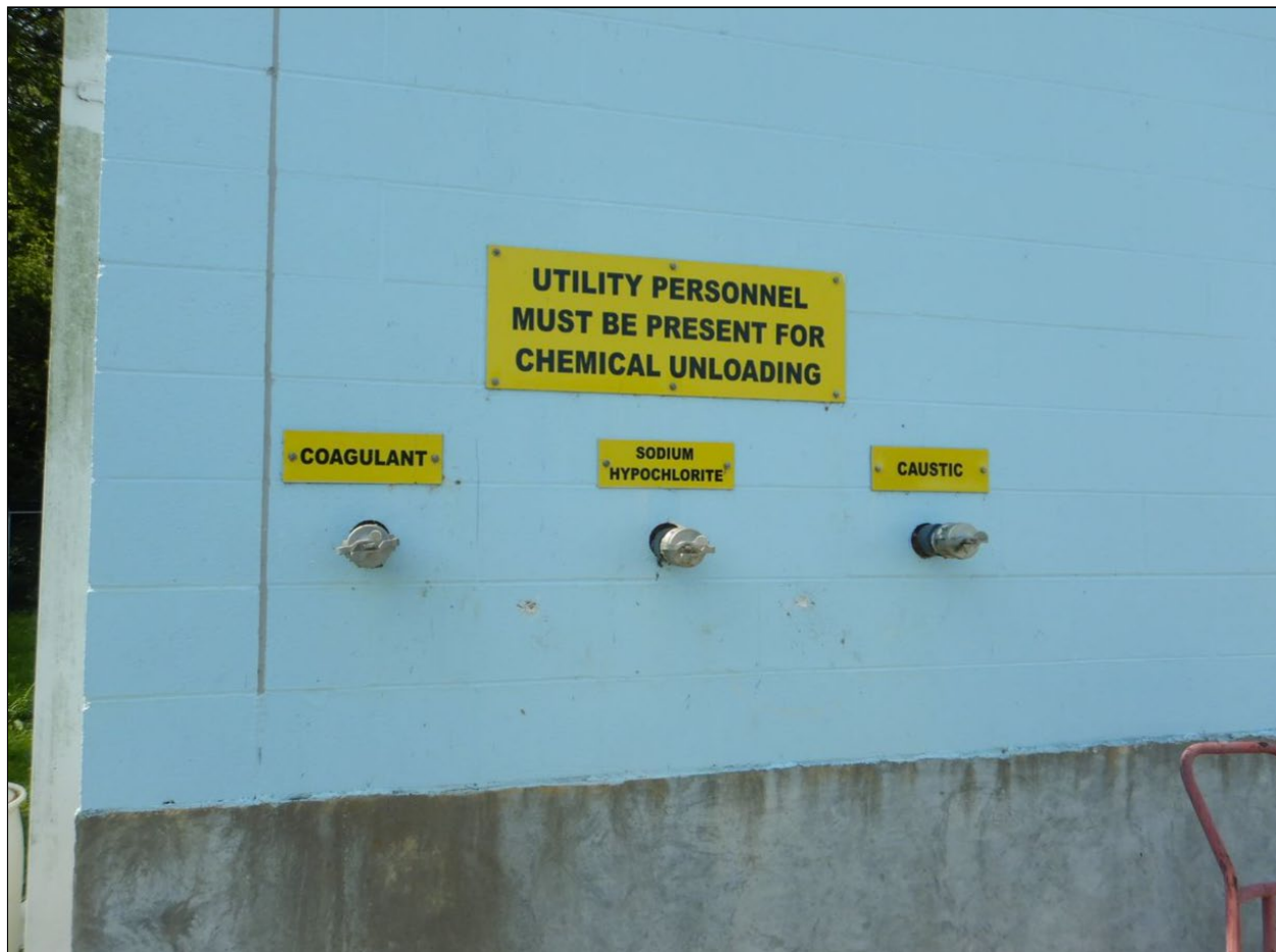
Photograph 6. Chemical Delivery Ports, WTP #01 View of the chemical delivery ports for coagulant, sodium hypochlorite, and caustic located on the exterior of the chemical storage area at WTP #01. System representatives stated that chemicals were sampled prior to being unloaded.
