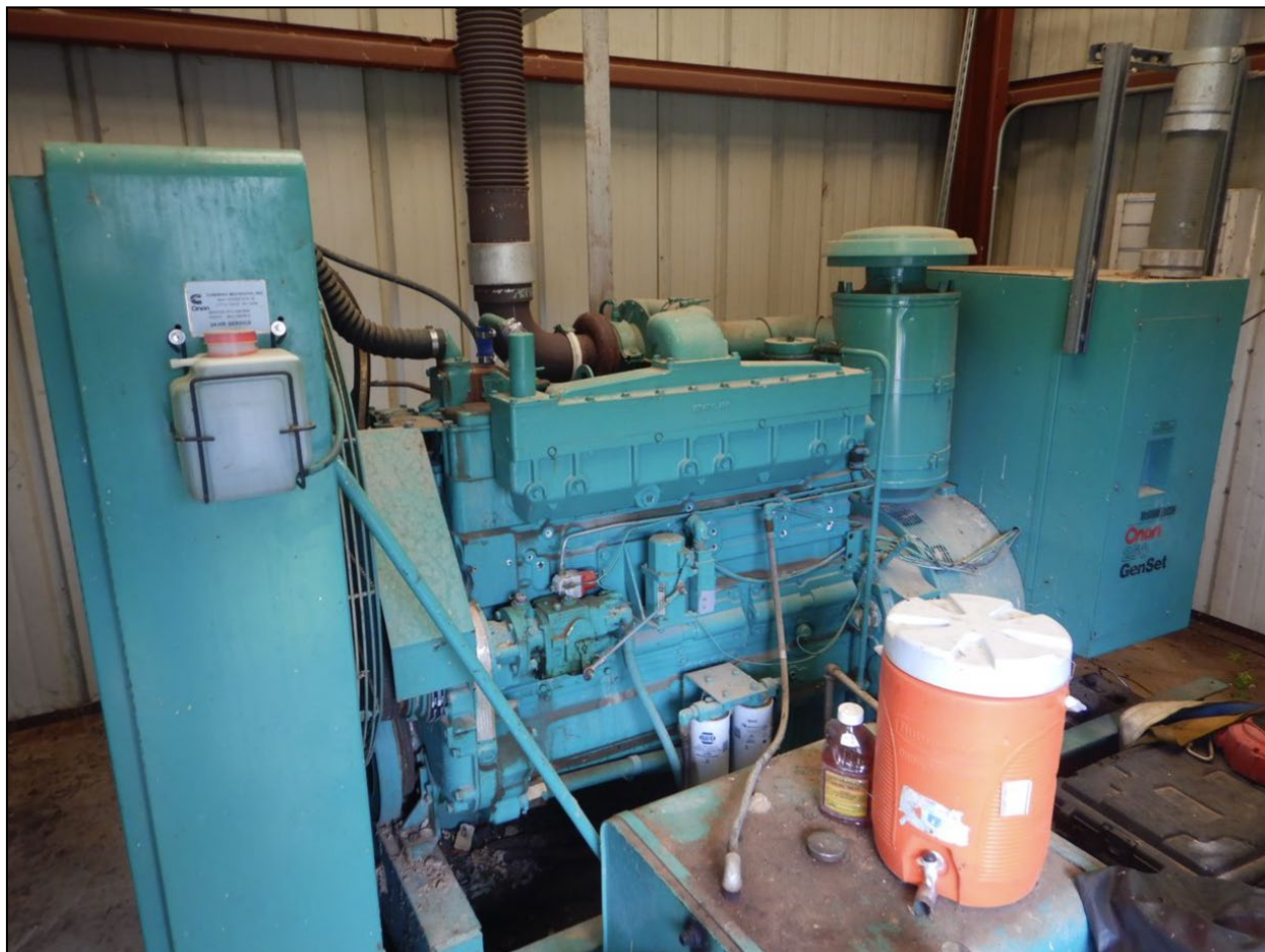
Photograph 9. Mounted Generator, WTP #01 View of one of the three onsite mounted generators at WTP #01. This was one of two generators that need to be turned on manually in the event of a power outage.
