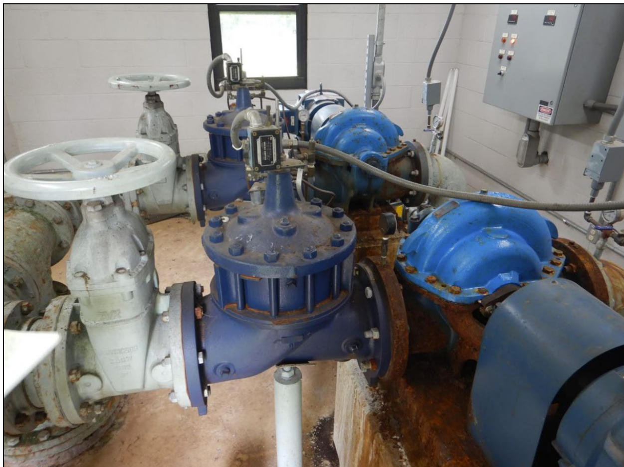
Photograph 33. 26 th St. Pump Station View of the inside of the 26 th St. Pump Station. The System Manager stated that the 26 th St. Water Storage Tank was filled by gravity, and that this pump station was used to send water to the Malone Water Storage Tank.
