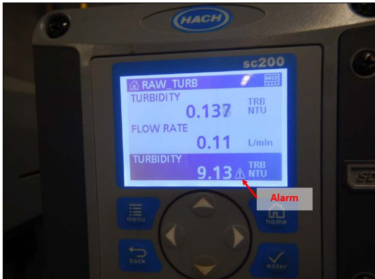
Photograph 15. Turbidity Meter, WTP #01 View of the raw water turbidimeter reading that was displaying 9.13 NTU with an alarm during the inspection. System representatives were unsure what was causing the alarm, but they assumed that the alarm was a result of a clogged raw water line leading to the turbidimeter.
