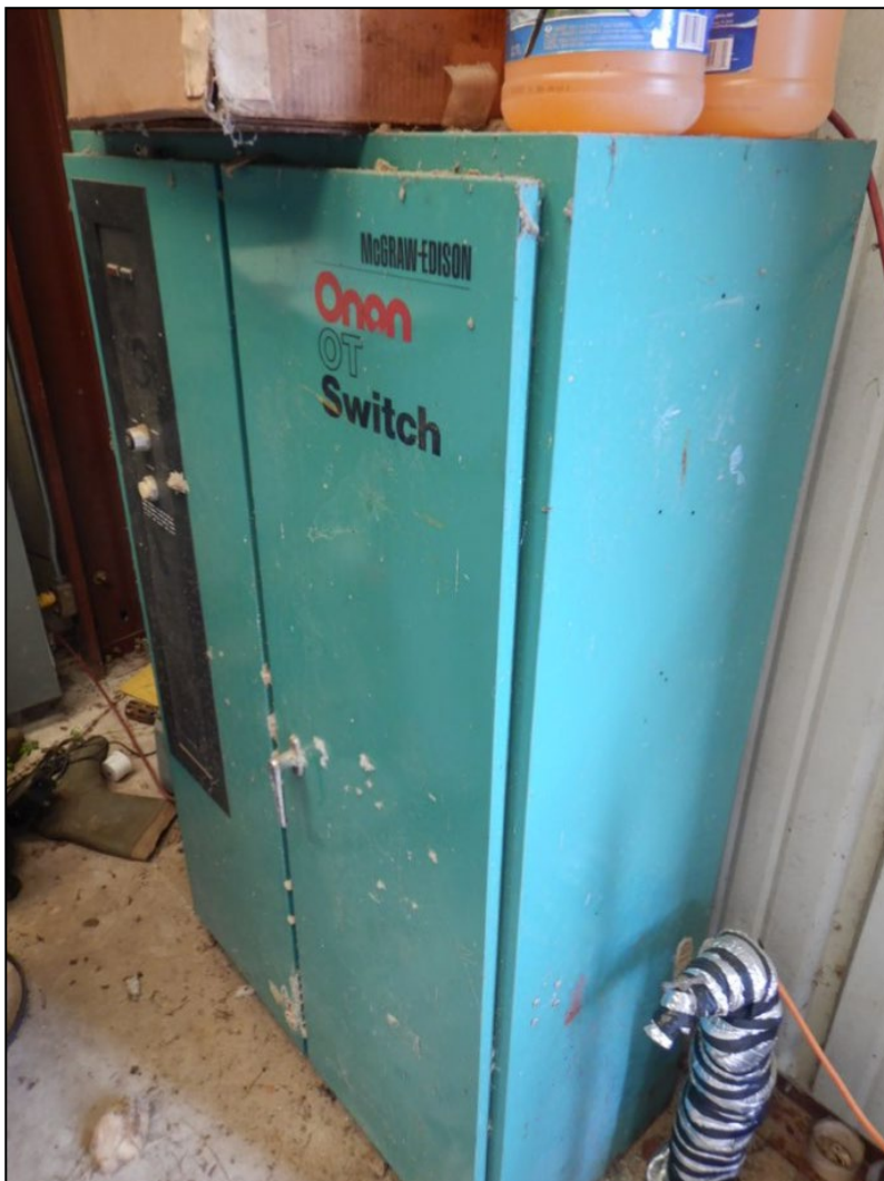
Photograph 11. Switch Gear Box View of an offline switch gear box associated with one of the two manual start up generators. The System Manager stated that this was not in use, but if it was functional could be used to turn on the backup generator automatically in the event of a power outage.
