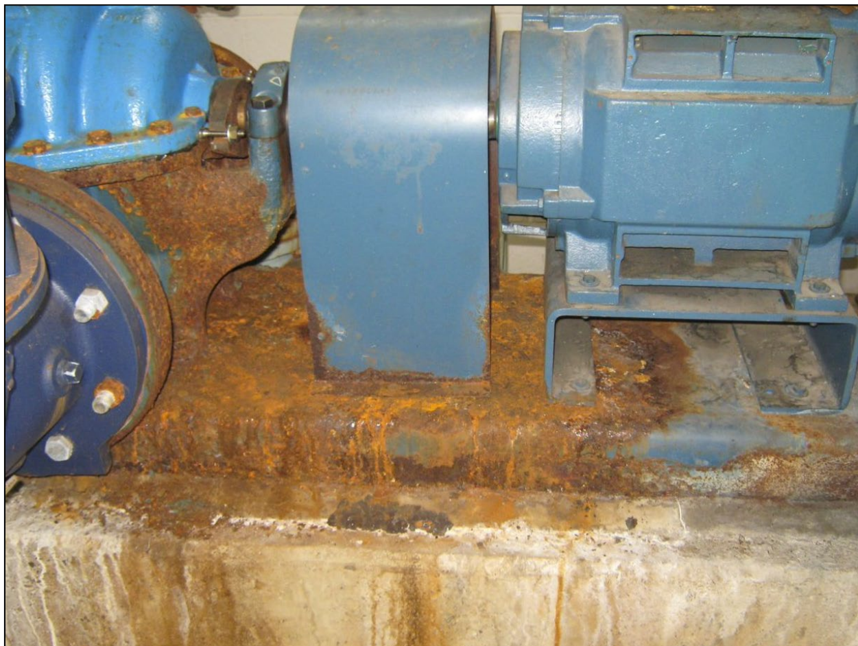
Photograph 34. 26 th St. Pump Station View of one of the pump mounts inside of the 26 th St. Pump Station that was experiencing corrosion/metal loss.
