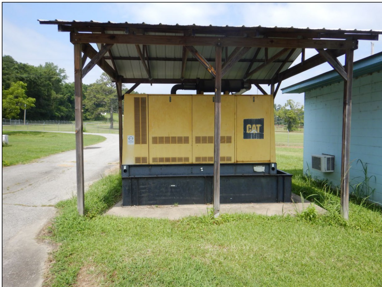
Photograph 10. Mounted Generator, WTP #01 View of one of the three onsite mounted generators at WTP #01. This was one of two generators that need to be turned on manually in the event of a power outage.
