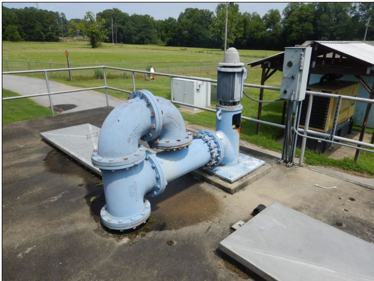
Photograph 20. Backwash Pump, WTP #01 View of the backwash pump and backwash holding tank that is used to send filtered (but not chlorinated) water through Filter Nos. 3-6. A separate backwash pump is used to send finished water from an onsite clear well through Filter Nos. 1 and 2.
