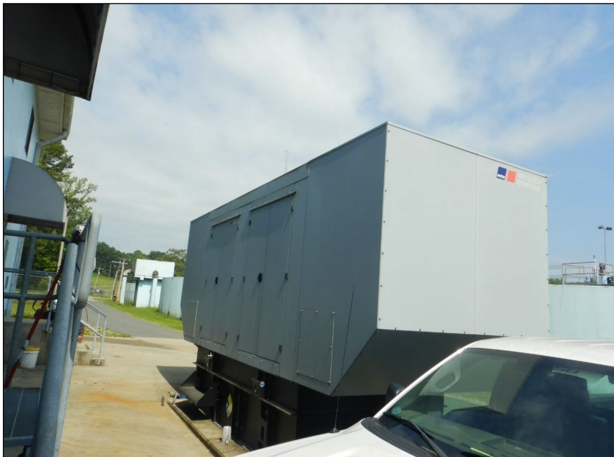
Photograph 8. Mounted Generator, WTP #01 View of one of three mounted backup generators at WTP #01. The System Manager stated that this was the only generator that would turn on in the event of a power outage.
