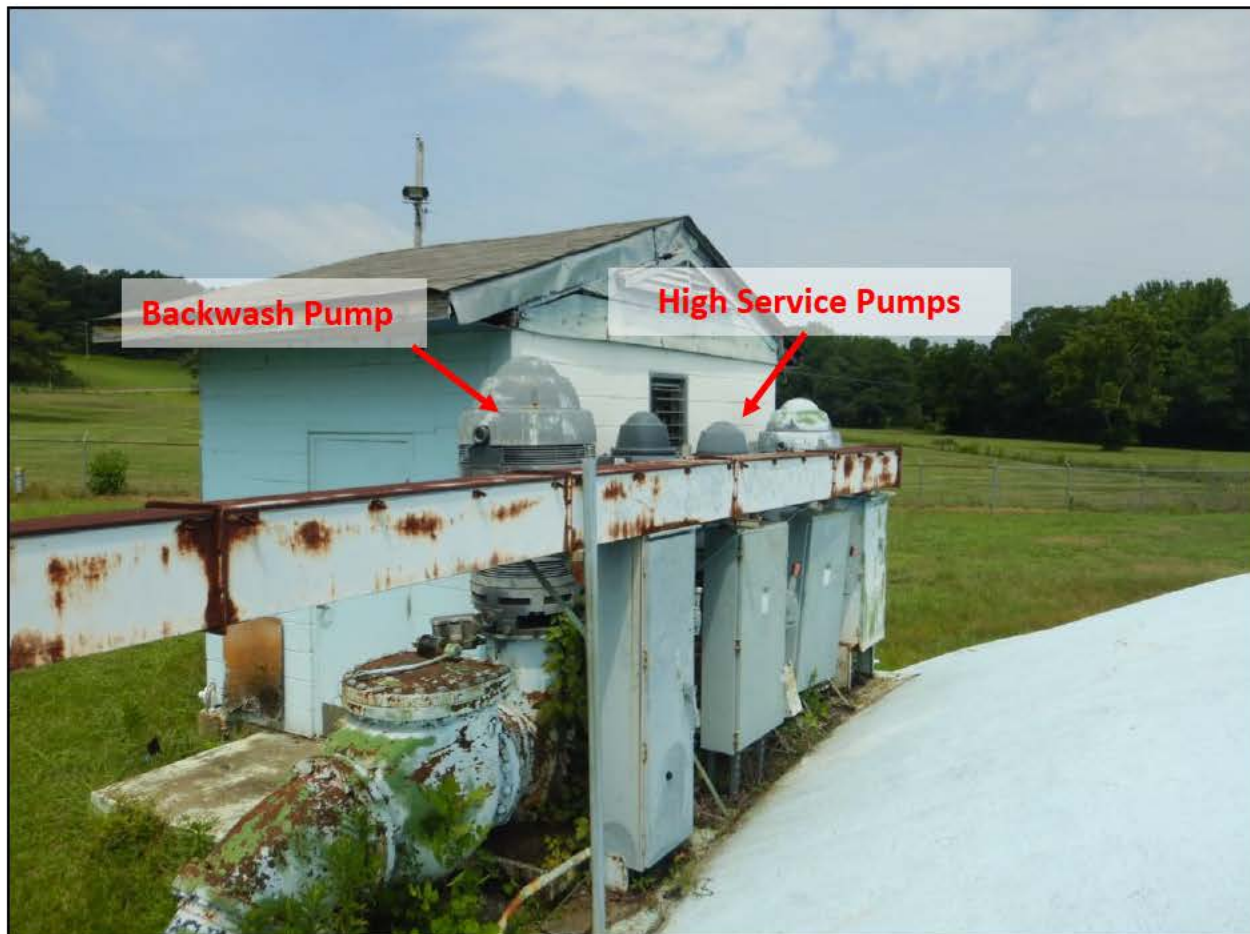
Photograph 22. Backwash Pump and High Service Pumps, WTP #01 View of the backwash pump used to send water from the clear well through Filter Nos. 1 and 2 during a backwash. Also visible are the three high service pumps used to send finished water into the distribution system.
